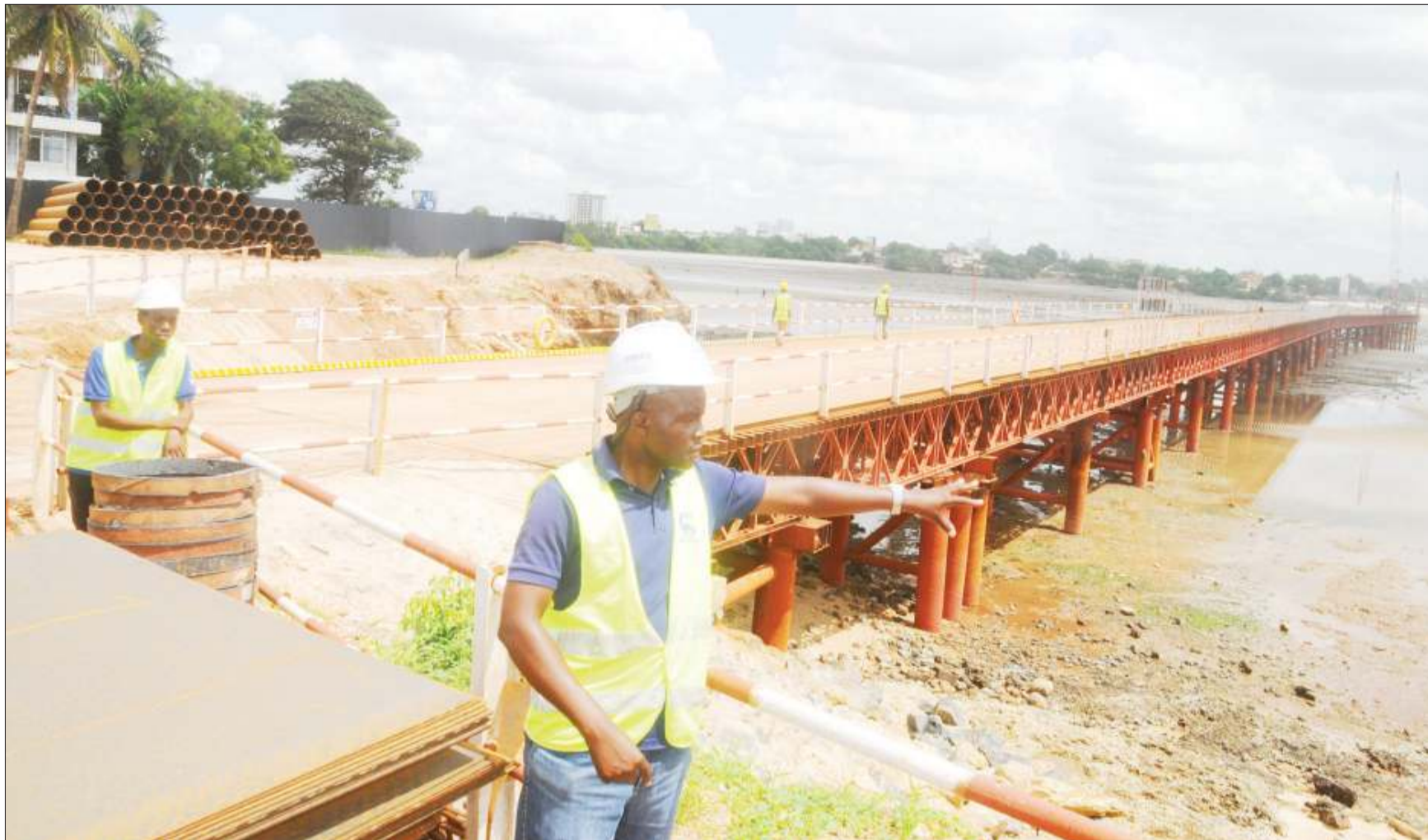
China Railway Major Bridges Engineering Group engineer Godwin Kambuga briefs journalists in Dar es Salaam yesterday on the ongoing construction of a temporary bridge in preparation for the implementation of the New Selander Bridge project. Left is the project's site engineer, Harepy Mrema. Photo: John Badi
