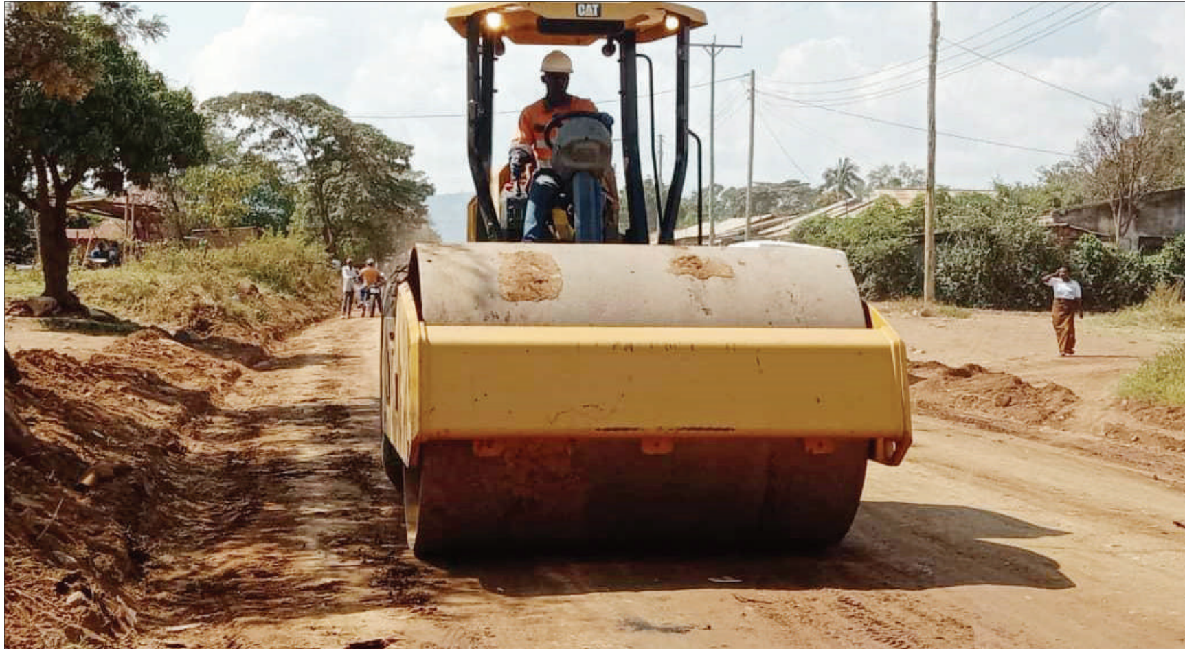
A grader repairs 3.6 Kilometers road linking Nyamongo and Kwanja townships in Tarime District in Mara Region. The project is being funded by Barrick Mining company. Photo: Guardian Correspondent
