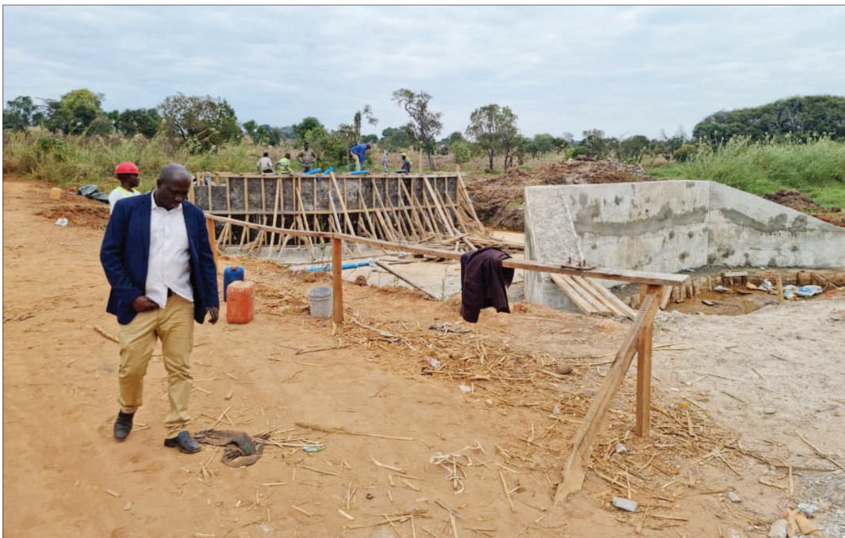
Tanzania Rural and Urban Road Agency Ruvuma regional manager Wahabu Nyamzungu inspects bridge construction connecting Madaba township and a health centre in Ruvuma Region over the weekend. Photo: Correspondent Gideon Mwakanosya
