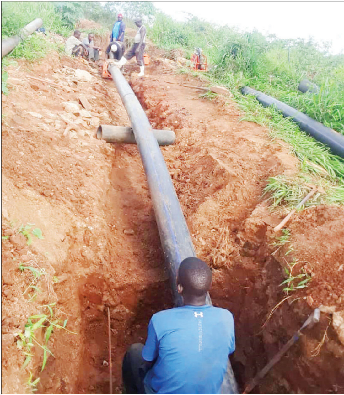
Dar es Salaam Water and Sanitation Authority technicians replace a water pipe at Mdaula in Coast Region yesterday to ensure better supply of tap water at Ubena, Mwidu, Visakazi villages as well as a nearby Army camp. Photo: Guardian Correspondent
