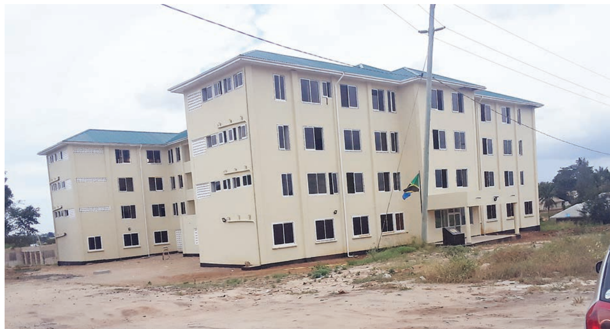
Mabwepande district hospital, Kinondoni Municipality, which was launched in February this year by President Samia Suluhu Hassani, when she was still the Vice President, in its completion stages. Photo: Correspondent Daniel Semberya.
