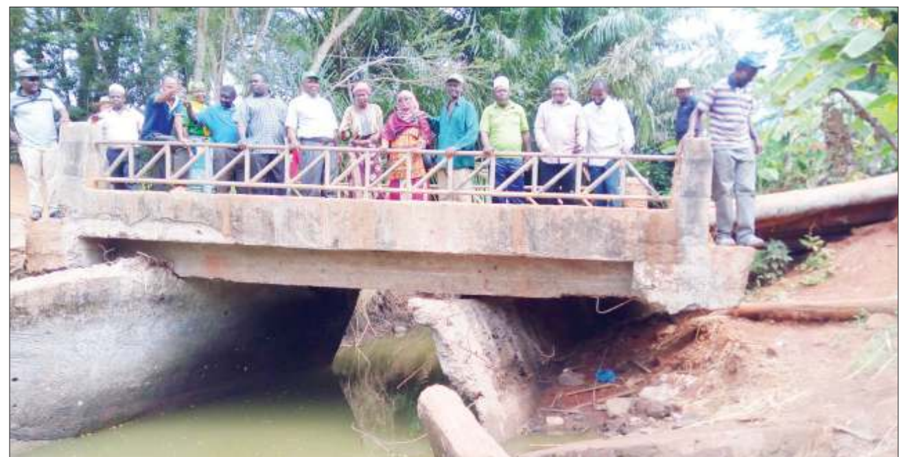
Muheza residents look at Bulunge river bridge which was washed away by floodwater last year. The bridge links Masuguru and Kerenge villages in Tanga Region. According to Tarura manager in Muheza the bridge will be rebuilt by a local contractor. Photo: Correspondent Steven William
