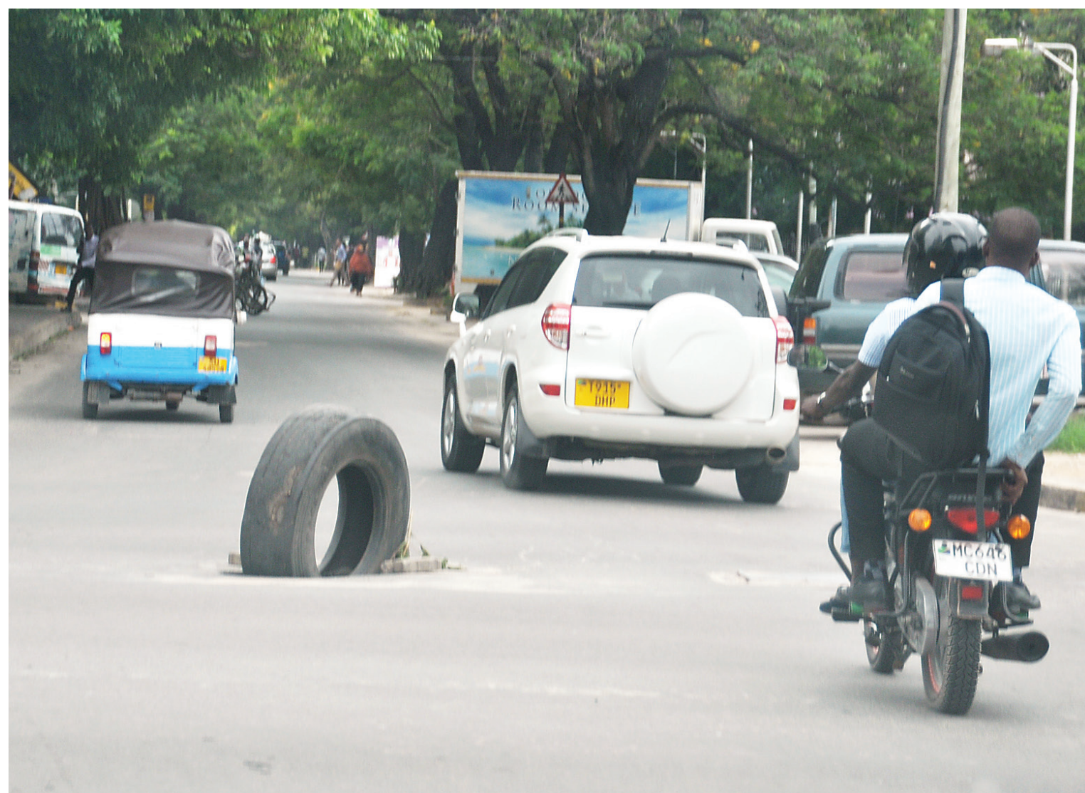
A used tyre 'deployed' at the Sokoine Drive/Azikiwe Street intersection in downtown Dar es Salaam serves to alert motorists on the need to steer clear of the pothole it partly covers, as found yesterday. Photo: John Babi
