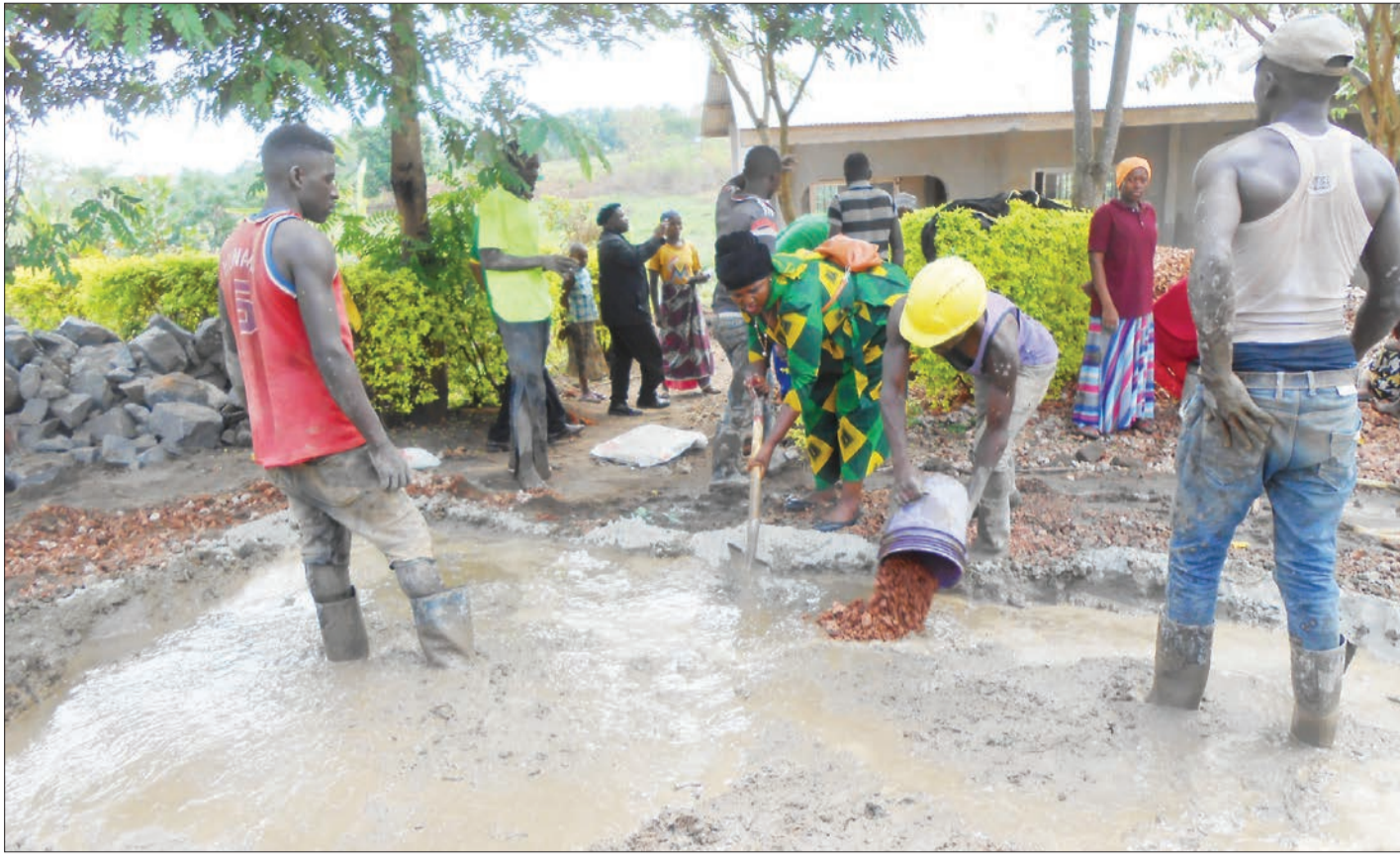
Habiba Mnguya (with shovel), Special Seats councillor for Kwekivu Division in Kilindi District, participates in construction work at Kilindi Asilia Secondary School yesterday. Photo: Correspondent Dege Masoli
