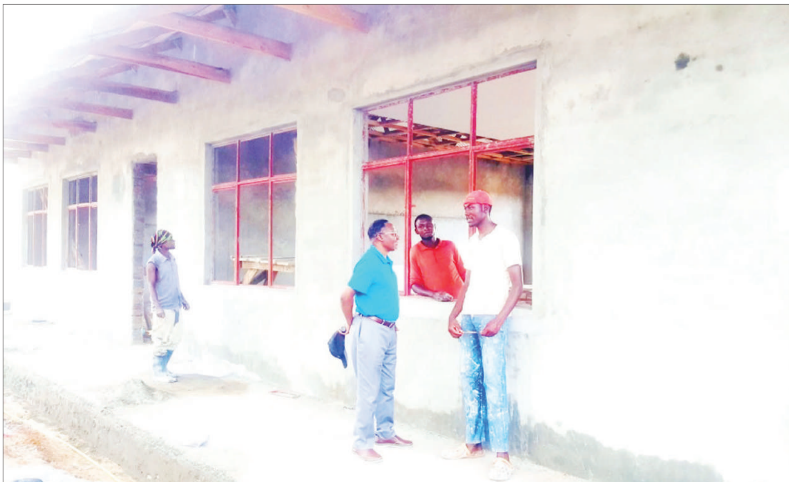
Journalists Environmental Association of Tanzania director John Chikomo (2nd R) talks to a mason working at a construction site at Burunge primary school in Manyara region recently. Photo: Correspondent: Aston Balaigwa
