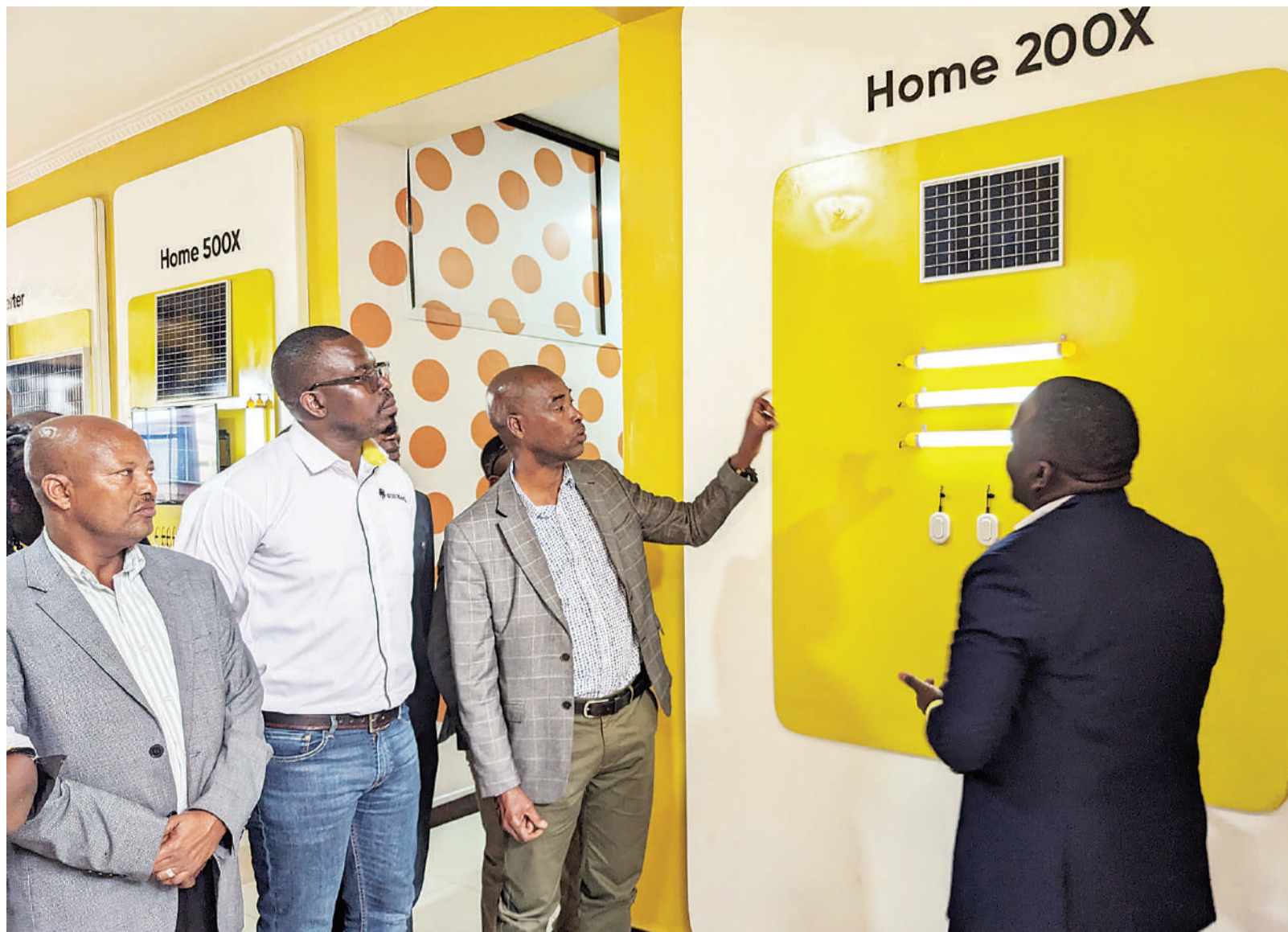
Arusha City mayor Maximilian Iranghe switches on solar inverter installed at the Themi Health Centre in Arusha at the weekend.
