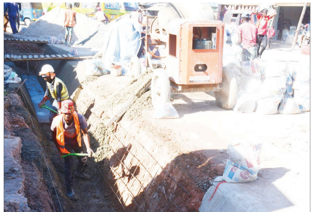
Construction of a sewage system well under way along a road in Dar es Salaam's Kitunda suburb yesterday. Photo: Correspondent Jumanne Juma
