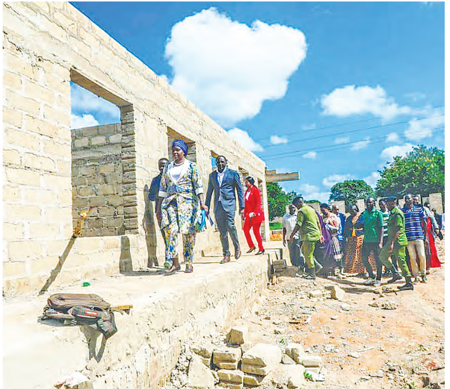
Dr. Dorothy Gwajima (L), Community Development, Gender, Women and Special Groups Minister, inspects construction of new primary school classrooms at Langoni area in Ulyankulu, Tabora Region, during her official visit to the region at the weekend. Photo: Guardian Correspondent.
