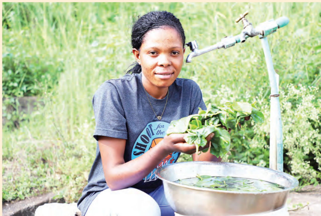
A resident washes vegetables with water provided by the Arusha new water supply system project undertaken by Power Construction Corporation of China, in Arusha, Tanzania, on Jan. 28, 2024. The water supply project includes laying over 620 km of steel pipelines, constructing 11 pools and connecting the water supply pipeline network to 48,000 households, according to PowerChina. (Xinhua/Hua Hongli)
