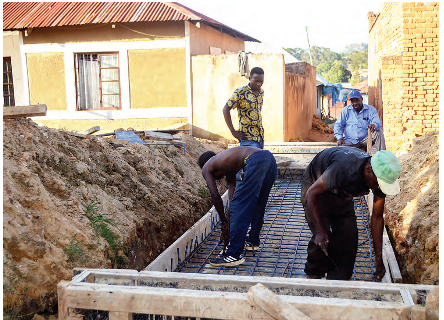
Construction of a culvert in progress on a road at Mwajombe in Kwakilosa ward, Iringa Municipality, as found yesterday. Photo: Correspondent Friday Simbaya
