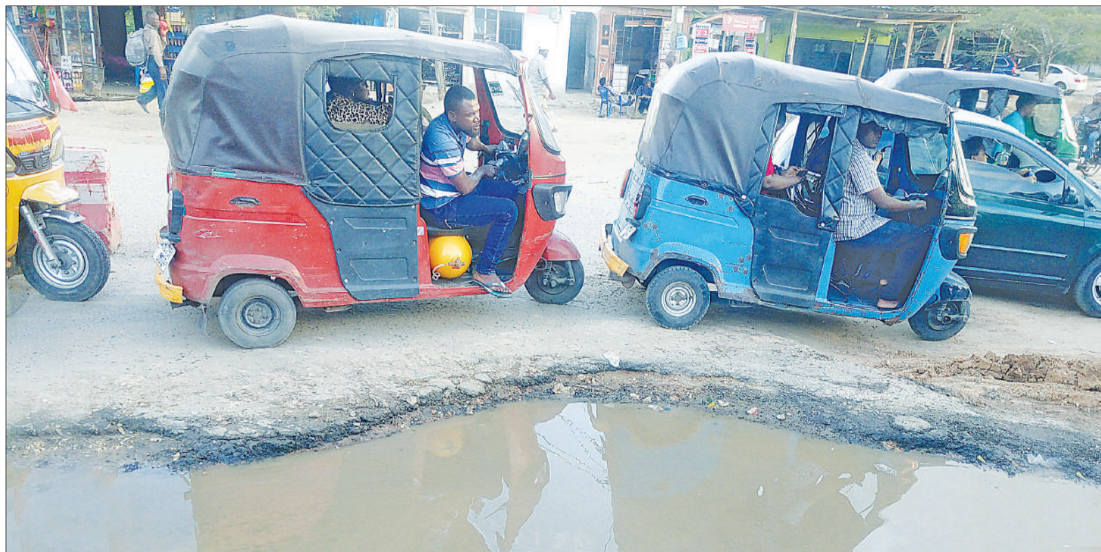
A gaping pothole-turned-pond forces motorists to move with caution along the Kimara Resort section of Morogoro Road on the outer reaches of the city on Monday, with a drizzle complicating the situation by blurring the edges of the pothole. Photo: Correspondent Sabato Kasika
