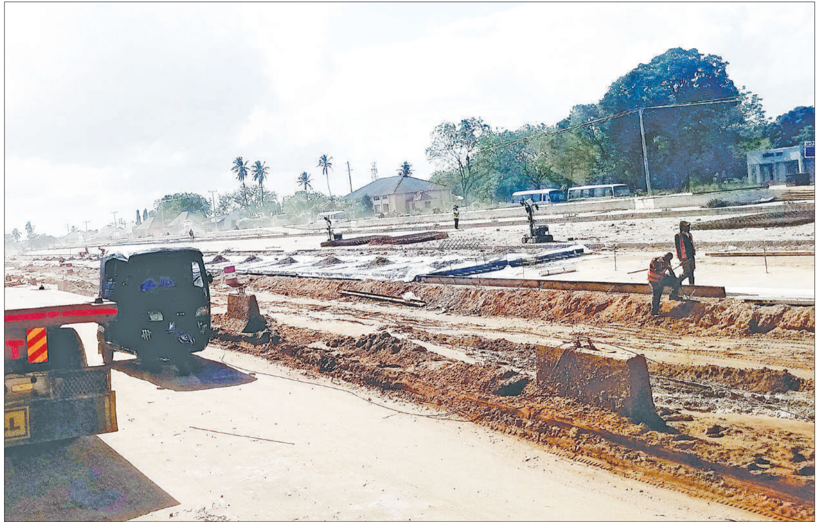
Construction of a rapid transit bus terminal at a section of the main road in progress Dar es Salaam's Gongo la Mboto suburb yesterday. Photo: Correspondent Sabato Kasika
