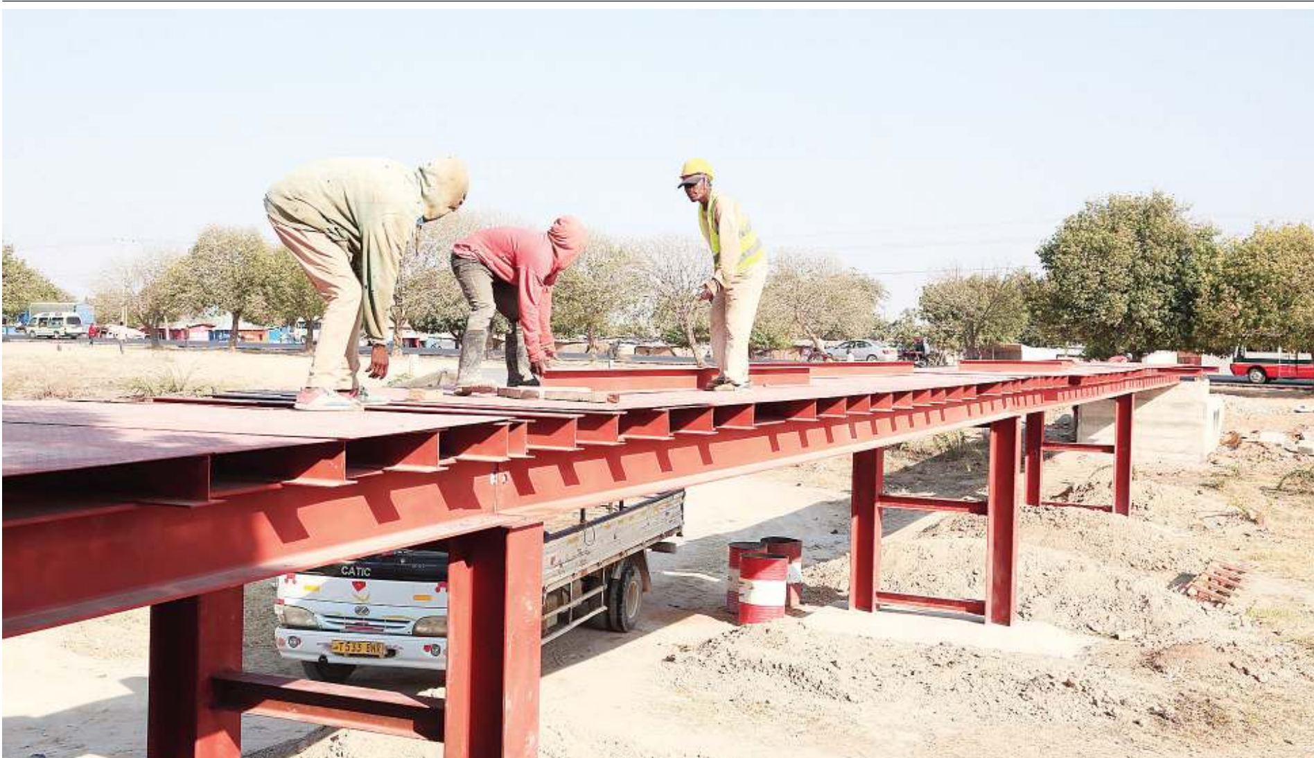
Construction of a pedestrian bridge well in progress at Chaduru B in Dodoma Region, as captured yesterday. The food-prone area gets hardly passable particularly during heavy rains. Photo: Correspondent Ibrahim Joseph
