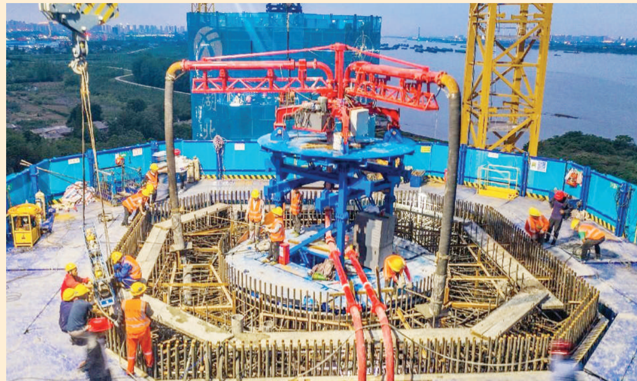
The main tower of the Yanji Yangtze River Bridge in Ezhou, central China's Hubei province, is being constructed. (Photo by Zhao Guangliang/People's Daily Online)
