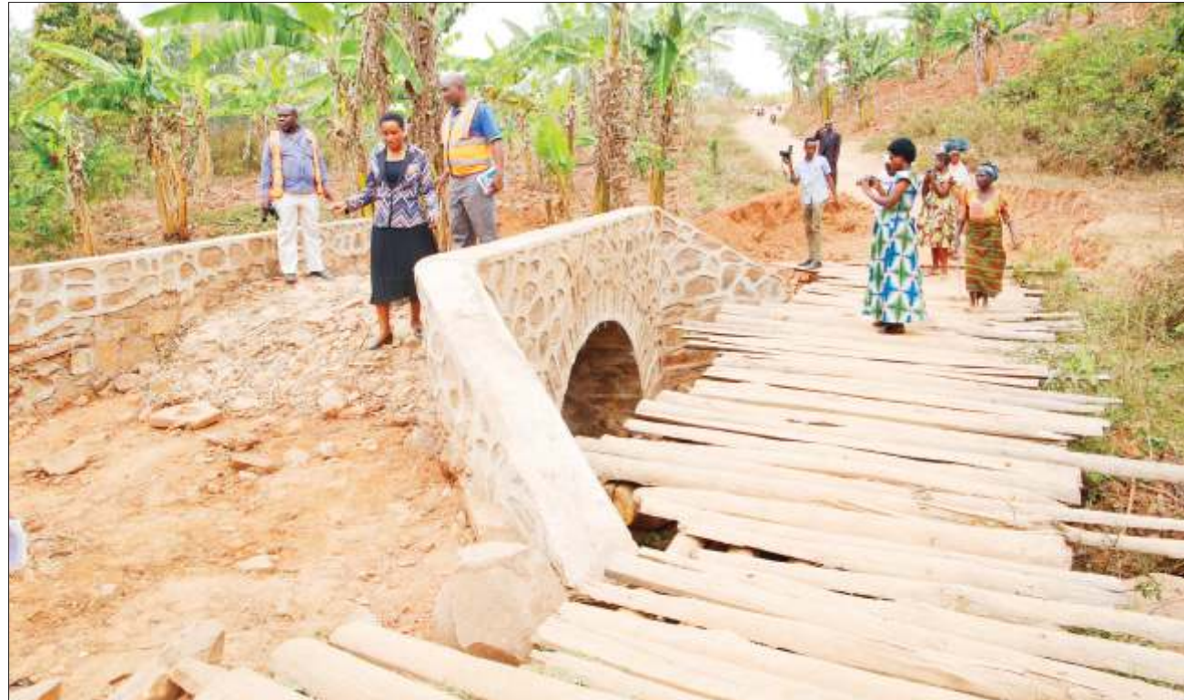
Kigoma district executive director Pendo Mangali (L, foreground) has a first-hand account of the ongoing construction of a bridge at Rubumba in Nyarubanda village yesterday. Others are Tanzania Rural and Urban Road Agency (Tarura) officials. Photo: Tarura
