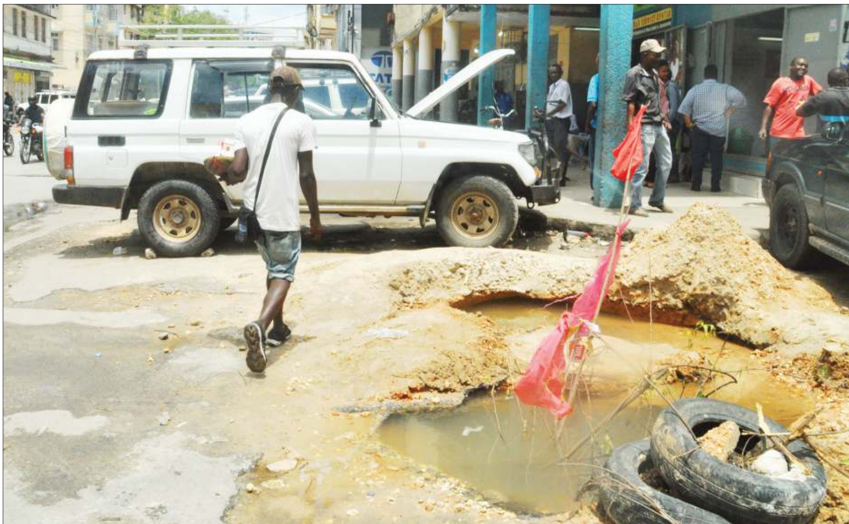
DANGER: A section of Libya Street in downtown Dar es Salaam has been all but rendered impassable for weeks now, what with the existence of the gaping pothole to the right, as found yesterday afternoon. Photo: John Badi
