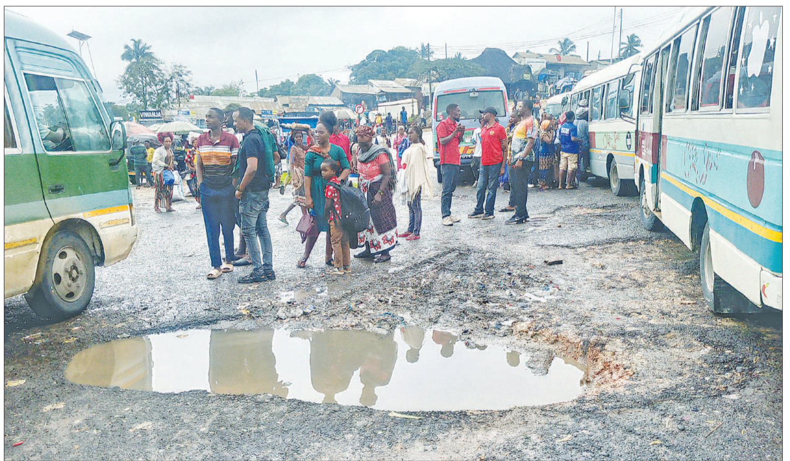
A gaping pothole at Dar es Salaam's Mbezi Mwisho commuter bus stand makes life especially hard for motorists, would-be passengers, disembarking passengers and passers-by, what with the incessant pounding rains in the city. Photo: Correspondent Sabato Kasika
