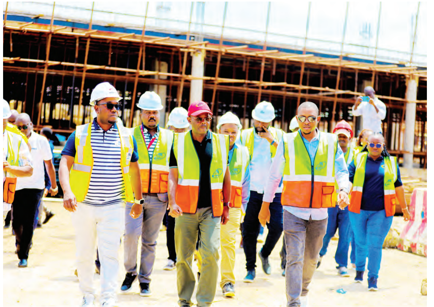
Transport Minister Prof Makame Mbalawa (with red cap) inspects progress of Mwanza South Port expansion project in Mwanza Region at the weekend. The port is expected to accommodate MV Mwanza "Hapa Kazi Tu" ship upon its completion in May this year. Photo: Vitus Audax
