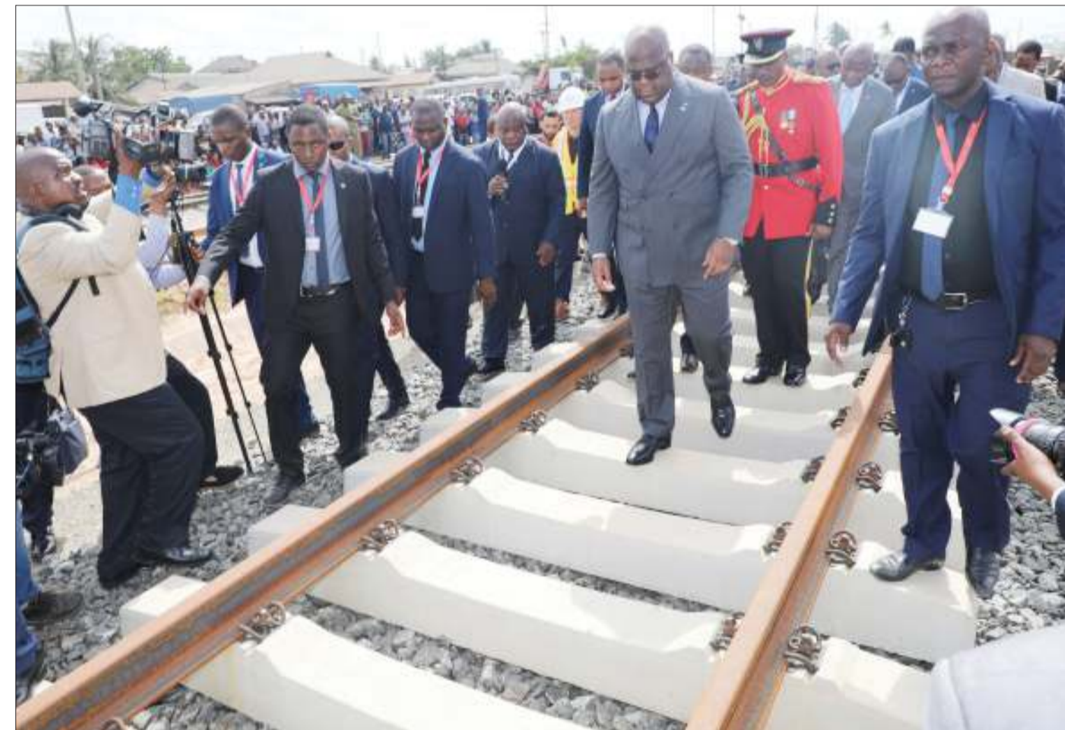
Democratic Republic of Congo President Félix Antoine Tshisekedi Tshilombo has a first-hand account of the ongoing implementation of the Standard Gauge Railway project by witnessing construction at Vingunguti in Dar es Salaam yesterday as part of his two-day state visit to Tanzania. . Photo: State House .
