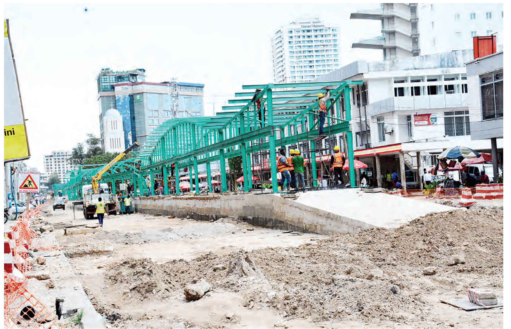
Construction of a Bus Rapid Transit station along Azikiwe Road in downtown Dar es Salaam in progress yesterday. Photo: Correspondent Miraji Msala
