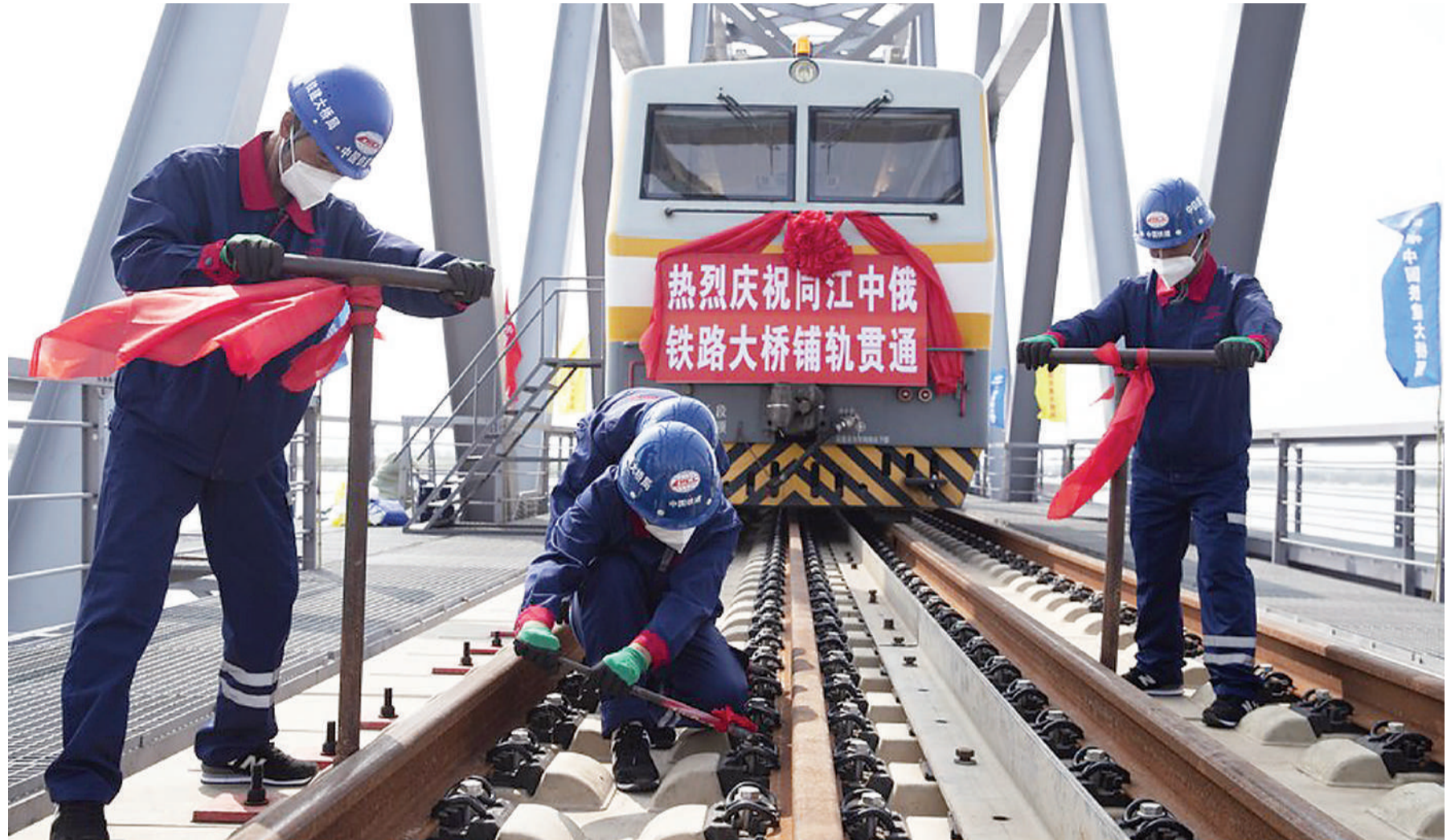
Constructors work at the construction site of the China-Russia Tongjiang-Nizhneleninskoye cross-border railway bridge, Aug. 17, 2021. (Xinhua/Zhang Tao)
