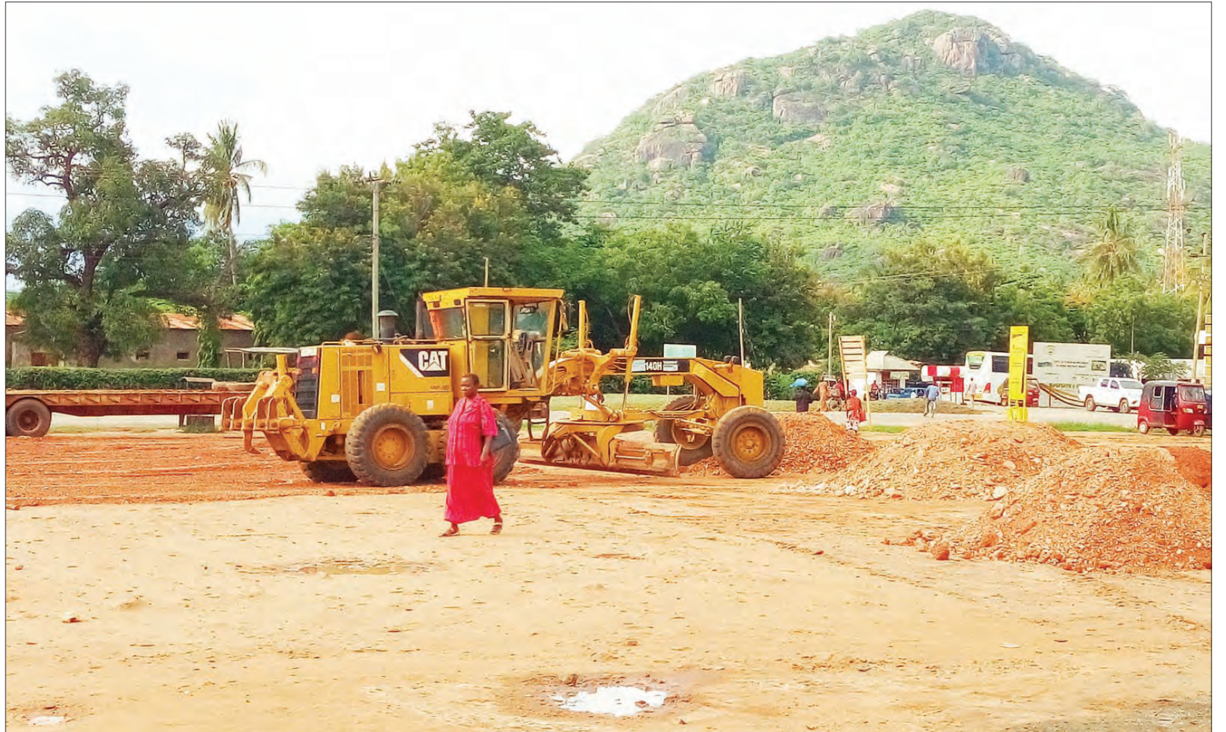
Caterpillar levels the ground surface at Masasi bus stand as part of rehabilitation efforts by the district council. Photo: Correspondent Hamisi Nasri
