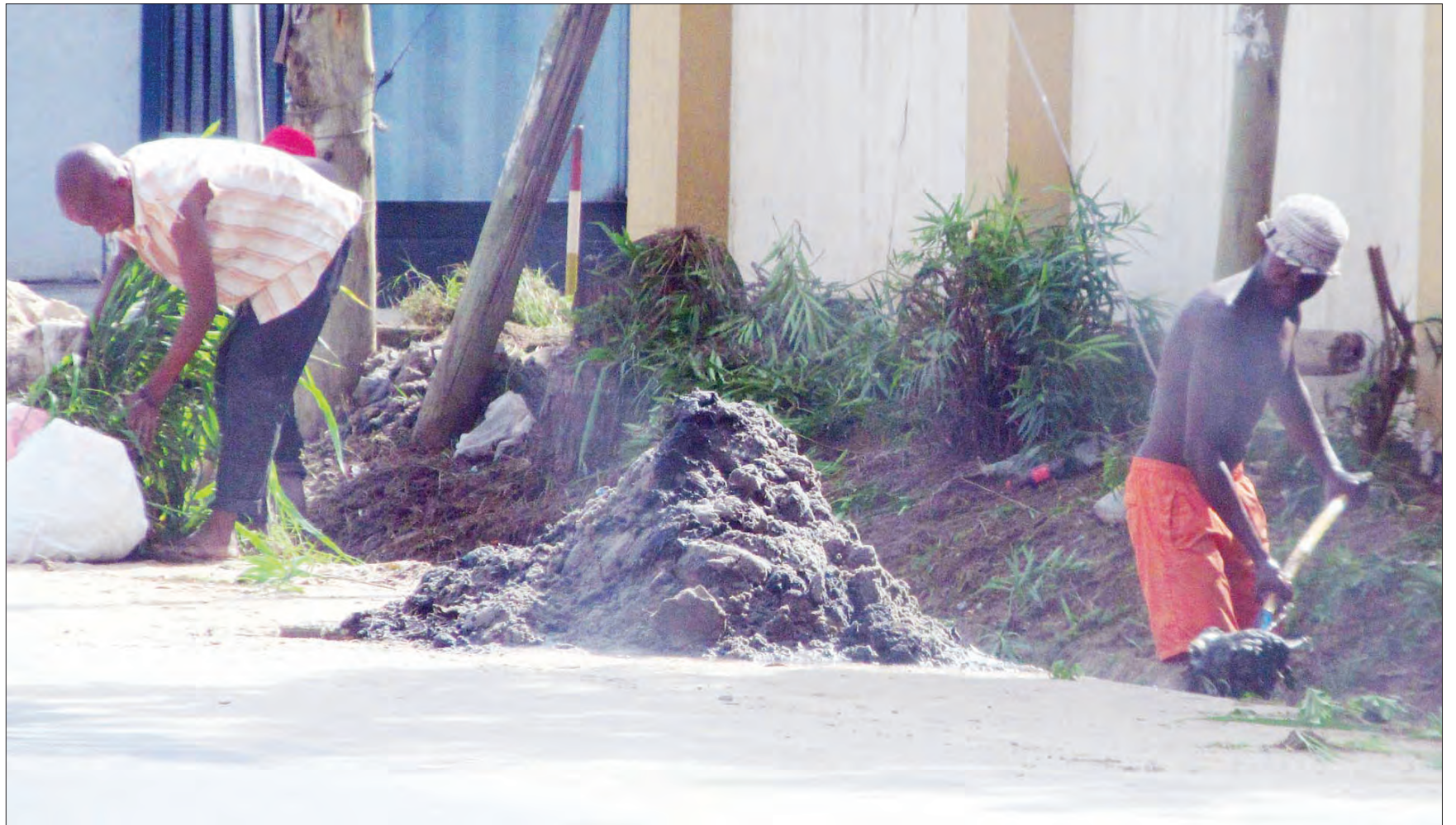
Following the ongoing rains some drainage system had been blocked. Mbezi Mwisho resident in the outskirts of Dar es Salaam clears mud to allow water flowing smoothly. Photo: Sabato Kasika
