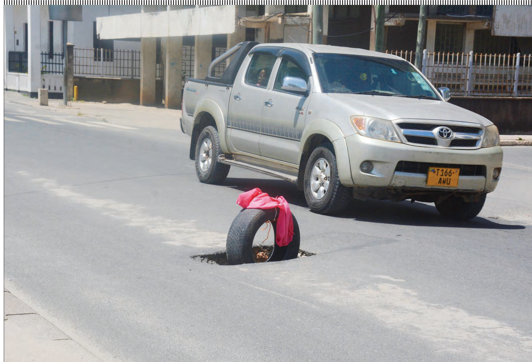
Precaution as motorists negotiate to avoid a hole along Sokoine Drive at Old Post Office in Dar es Salaam yesterday. Photo: Correspondent Jumanne Juma.
