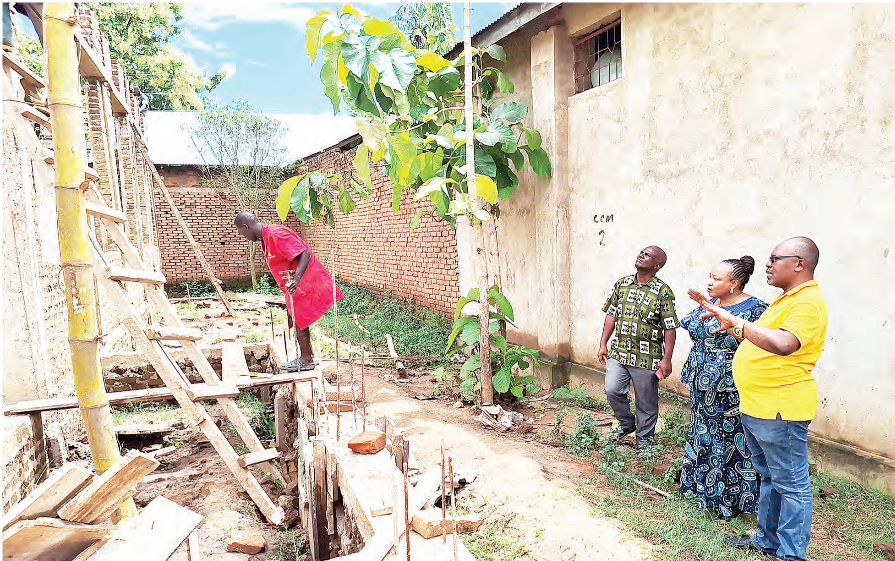
Joseph Mwambeleko (R), an official with CCM in Kilombero District, briefs the chairperson of the party's parents' wing for Morogoro Region, Dr Rose Rwakatare (next to him), on Thursday on progress in the ongoing construction of a building meant for the party's district office. Third right is the district's CCM chairman, Mohamed Msuya. Photo: Correspondent Joseph Mwendapole
