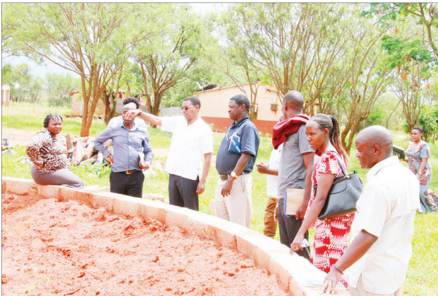
Sebastian Kitiku (3rd-L), an assistant director in the Health, Community Development, Gender, Elderly and Children, inspects the construction of a community centre at Kibaigwa Primary School in Dodoma Region yesterday. Photo: Guardian Correspondent
