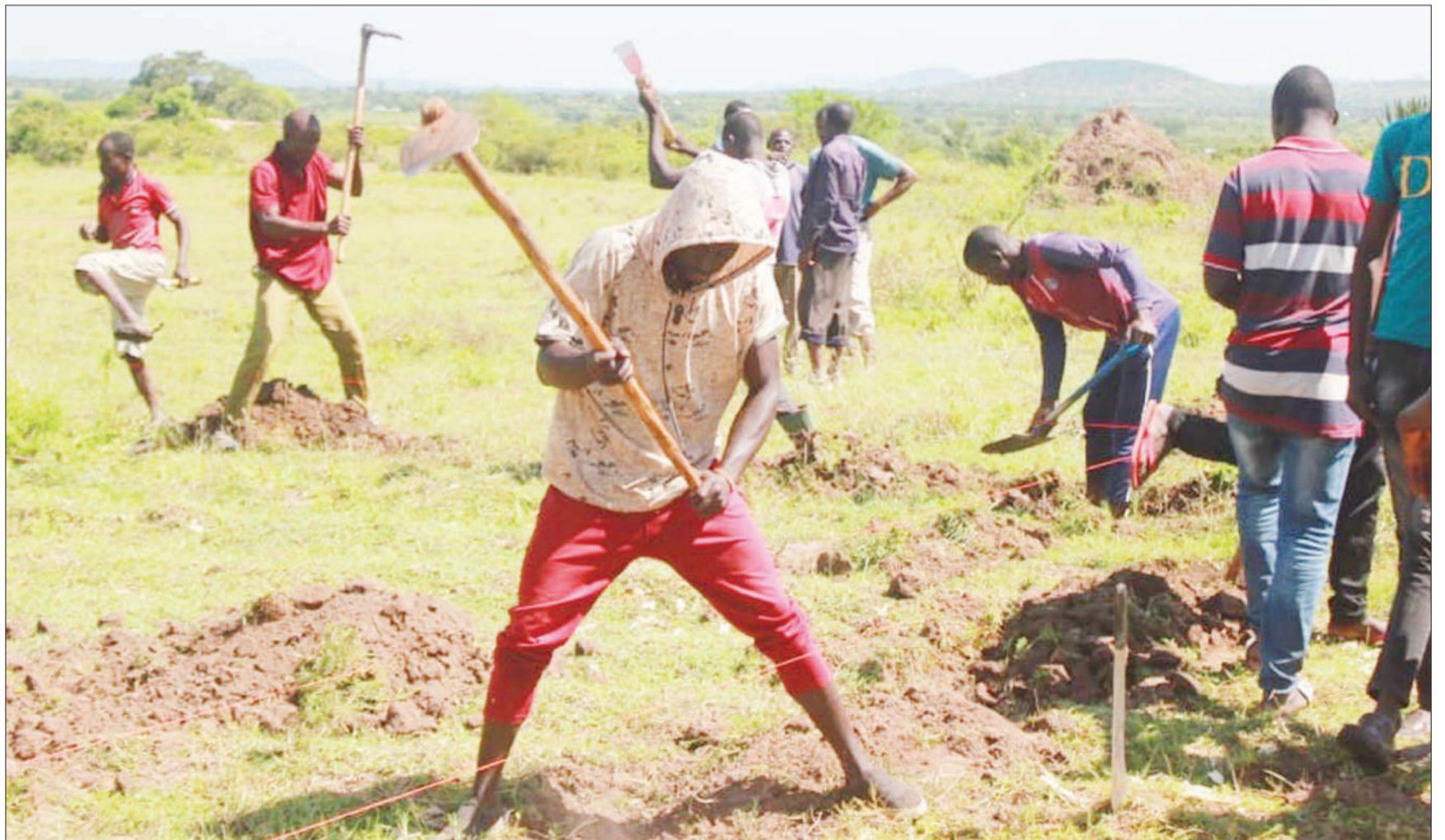
Rorya district commissioner Juma Chihoka leads the residents to dig the foundation stone for the construction of Rabuur health centre in Mara region over the weekend. Photo: Correspondent Samson Chacha
