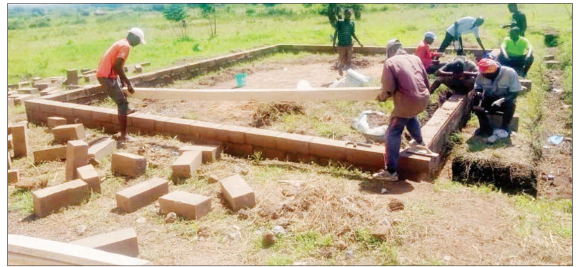
Masons busy with the construction of classrooms meant to accommodate the upcoming first intake of Form One students at Kigera Secondary School in the Musoma Rural constituency, as captured at the weekend. Photo: Guardian Correspondent
