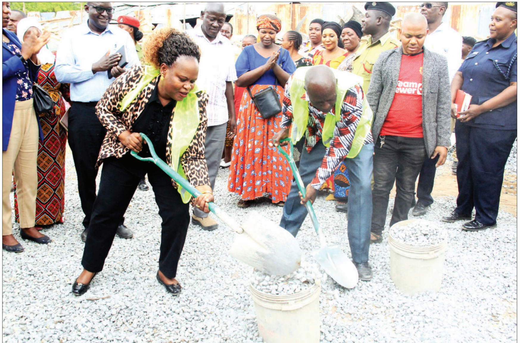
Shinyanga regional commissioner Christina Mndeme (L) and Shinyanga Municipal mayor Elias Masumbuko lend a hand in the construction of the municipal's main market during an inspection tour of progress in the implementation of the project on Monday. Photo: Correspondent Marco Maduhu
