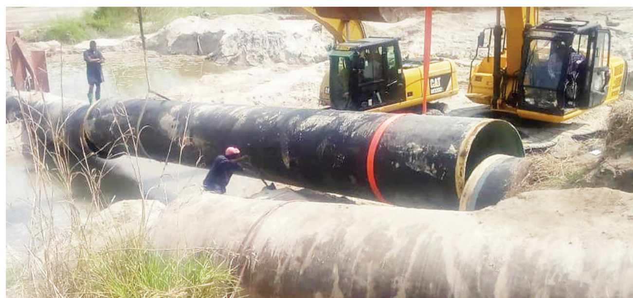
Dar es Salaam Water and Sanitation Authority (Dawasa) technicians move to re-install a water pipe swept away by heavy rains earlier this year, as found yesterday at Bunju on the outskirts of the city. Photo: Guardian Correspondent
