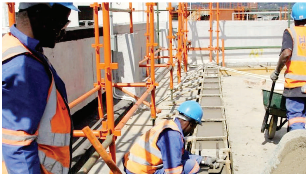
Construction mafias have been rife in KwaZulu-Natal over the past few years
