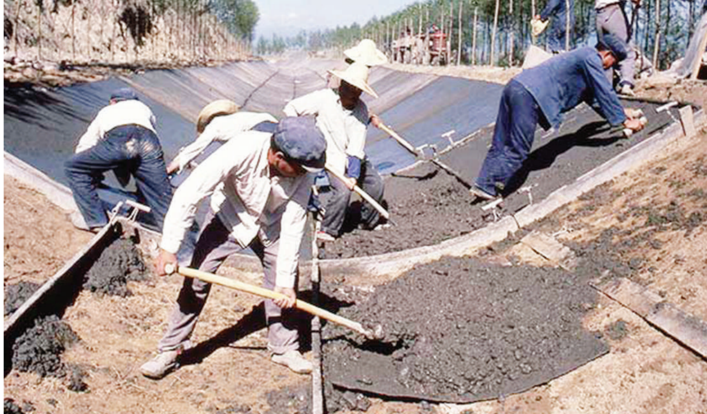
CHINA - Constructing an irrigation network in Qinghai Province. Workers were paid part of their wages in food supplied by the World Food Programme. Credit WFP/Sarah Errington
