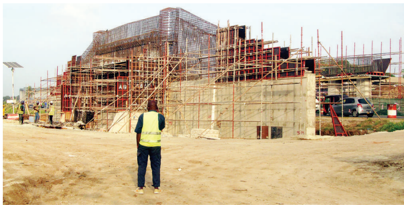
This is the stage the construction of a flyover along the Mbezi Mwisho section of Dar es Salaam's Morogoro Road has reached, as captured yesterday. Photo: Correspondent Sabato Kasika
