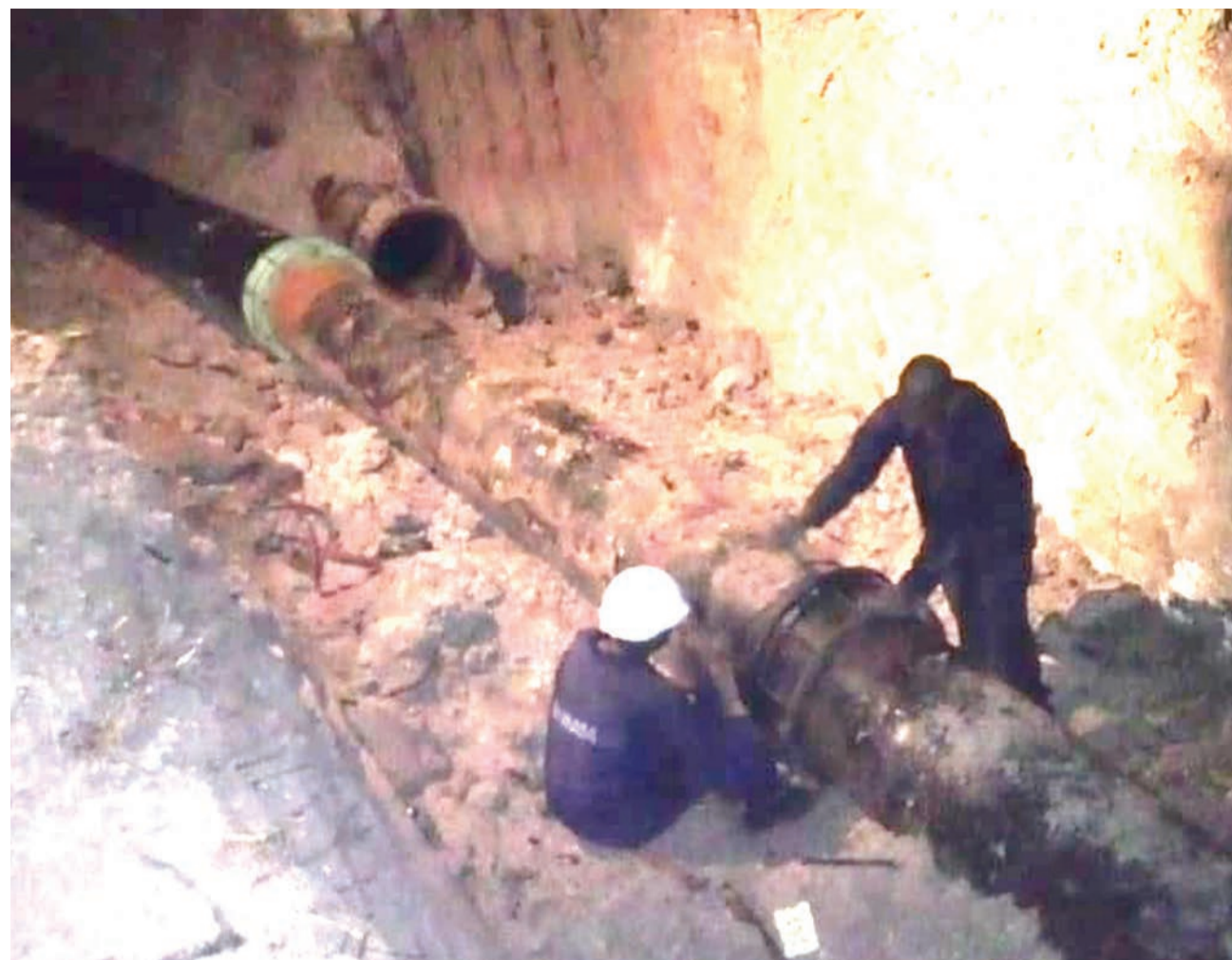
Dar es Salaam Water and Sewage Authority technicians remove a 24-inch pipe at Kibamba-Darajani on Wednesday to pave the way for the expansion of Morogoro Road. It was not immediately established whether this was behind the erratic nature of the supply of water parts of the city have been experiencing in recent days. Photo: Guardian Correspondent
