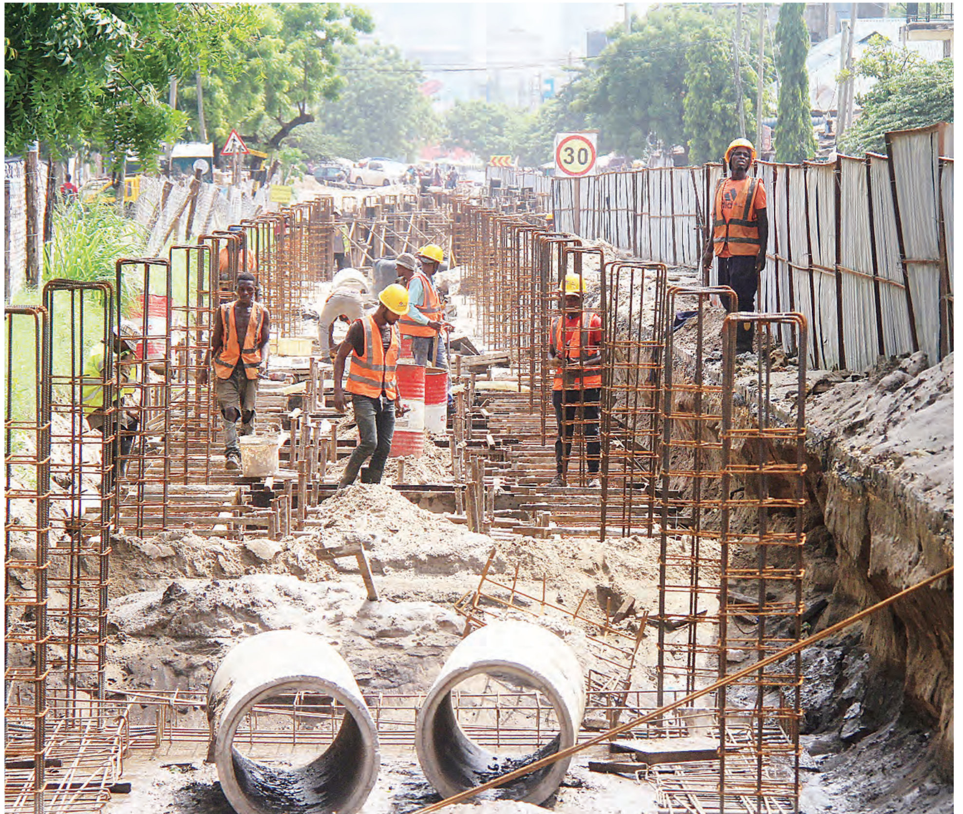
Work on Dar es Salaam's Bus Rapid Transit infrastructure in progress, as captured yesterday at the Ilala-Amama section of Uhuru Street. Photo: Correspondent Jumanne Juma
