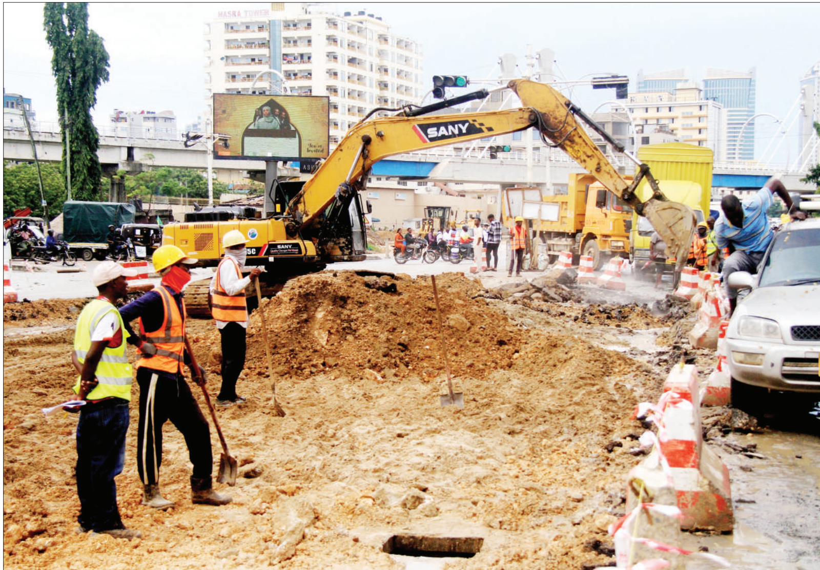
Preparations for the implementation of Phase II of the Dar es Salaam Bus Rapid Transit infrastructure project in progress along the Kamata stretch of Nyerere Road yesterday. Photo: Correspondent Jumanne Juma
