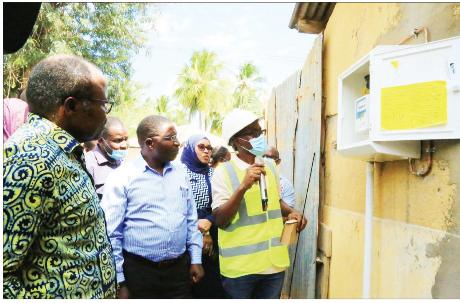
A Tanzania Petroleum Development Corporation expert (R) briefs Energy minister Dr Medard Kalemani (C, foreground) at Mnazi Mmoja in Lindi Region at the weekend on how natural gas meters installed in houses work. This was during the inauguration of the installation of natural gas infrastructure in houses in Lindi Region over the weekend. Left is Lindi Regional Commissioner Godfrey Zambi. Photo: Guardian Correspondent
