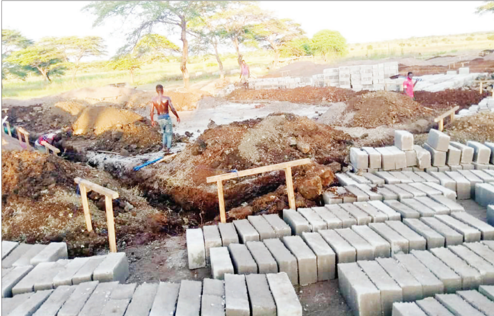
Masons work on the foundation of a building at Musoma Rural constituency's Masinono village dispensary, which is undergoing expansion - with the government having recently injected 400m/- into the project. The Guardian captured the scene at the weekend. Photo: Guardian Correspondent
