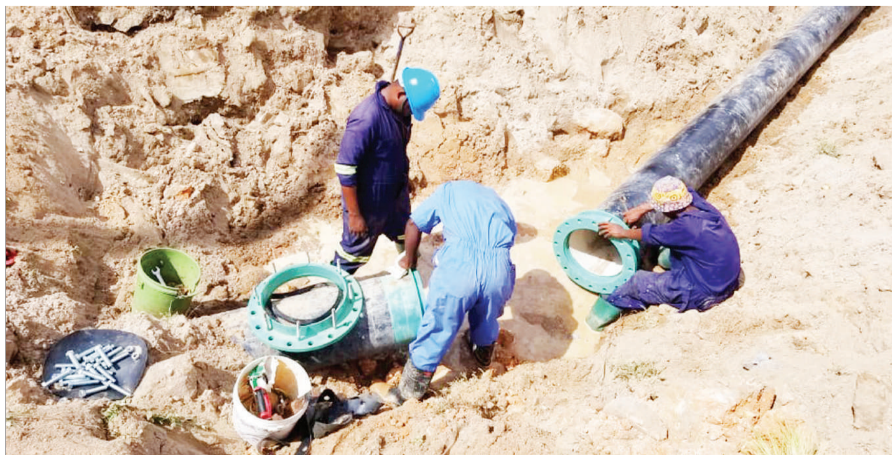
Dar es Salaam Water and Sanitation Authority (Dawasa) technicians connect a major pipe in the city's Buza suburb, with a view to making the precious liquid reach more people by later this week. Photo: Guardian Correspondent
