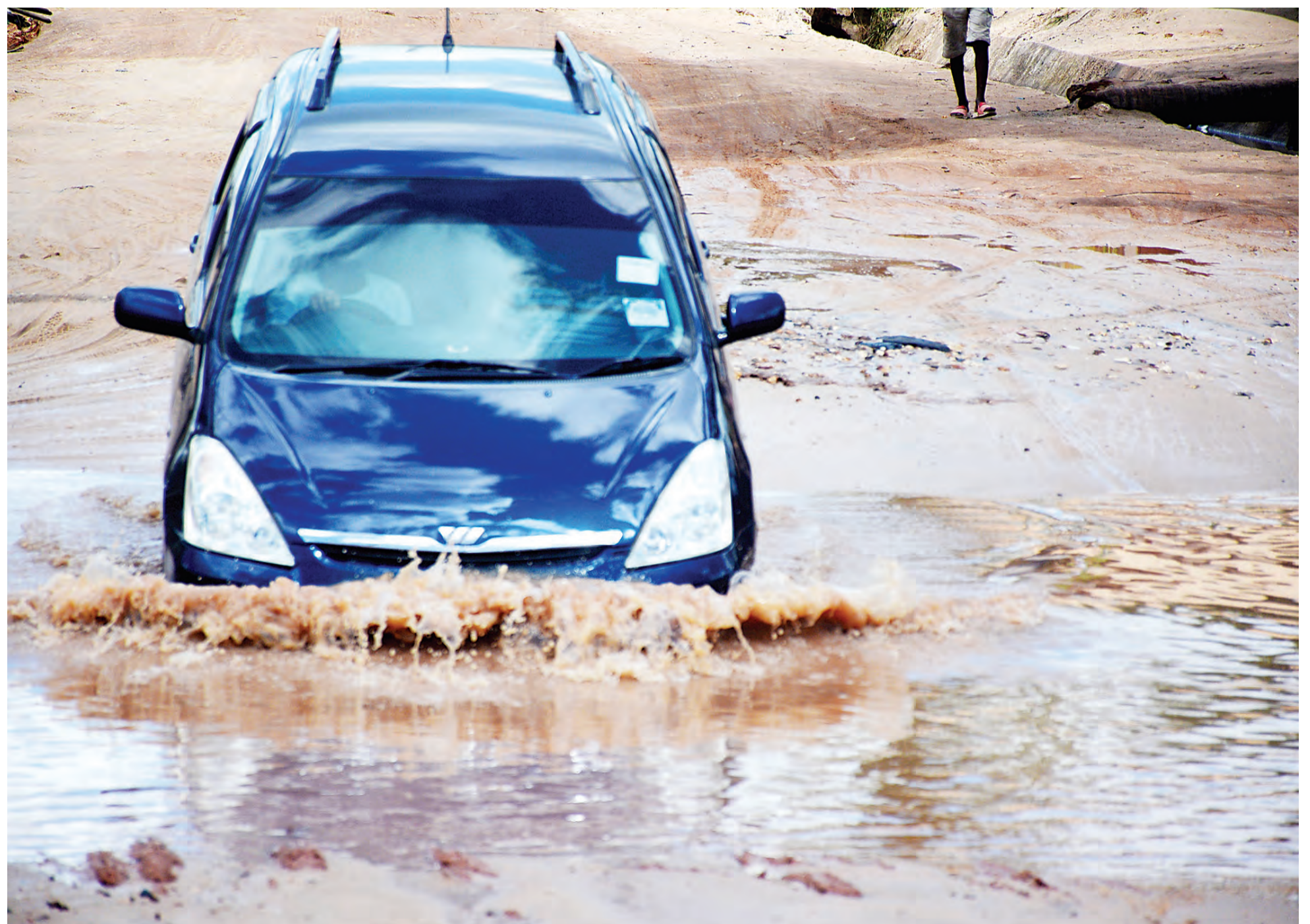
A motorist moves across a pond along a damaged section of a road at Msanga Zalala in Dar es Salaam's Chanika suburb earlier this week. Photo: Correspondent Jumanne Juma
