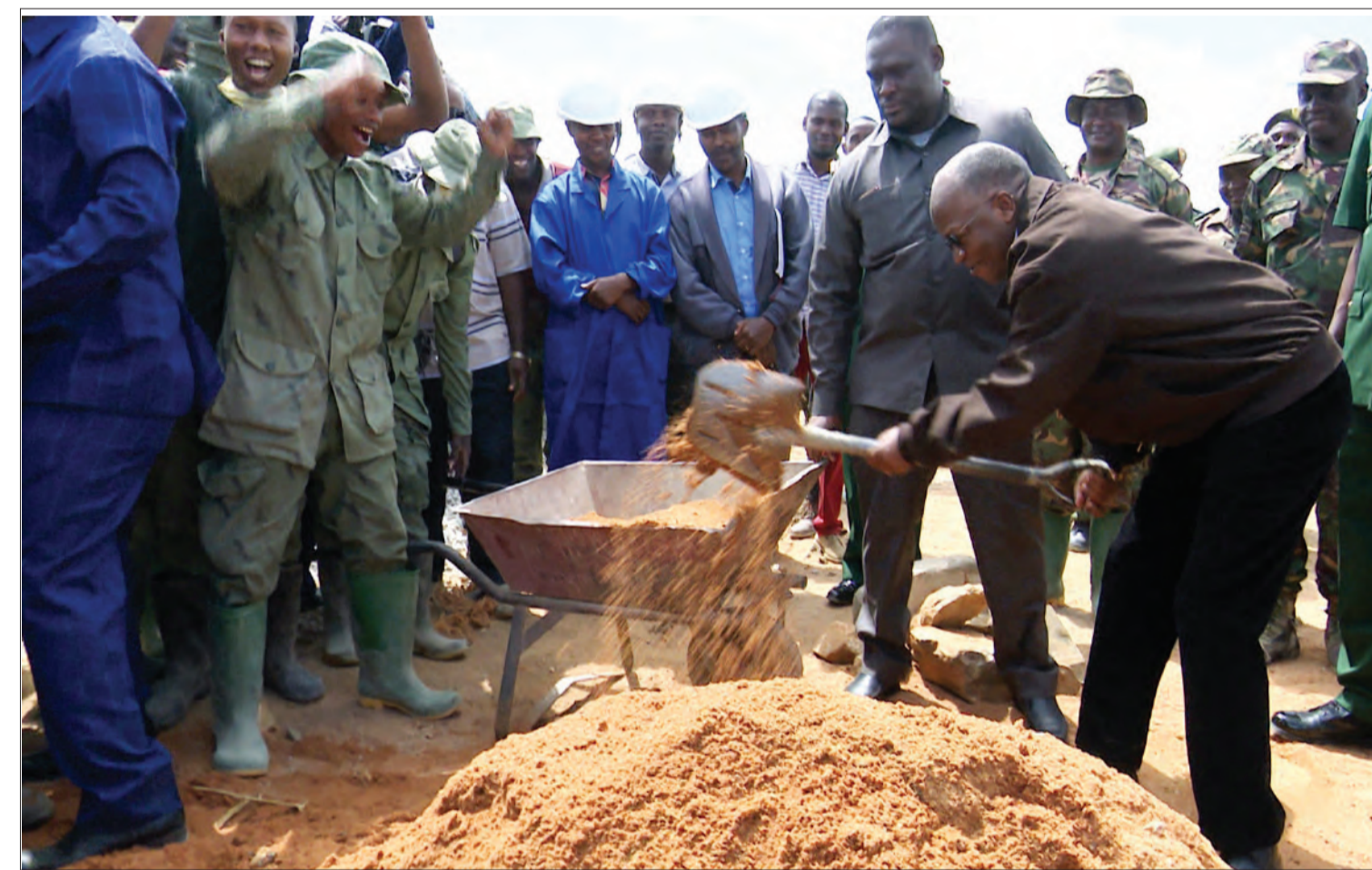
President John Magufuli chips in yesterday as preparations for the construction of an office building at Chamwino State House in suburban Dodoma got under way yesterday. He was on a routine tour of the project. Photo: State House
