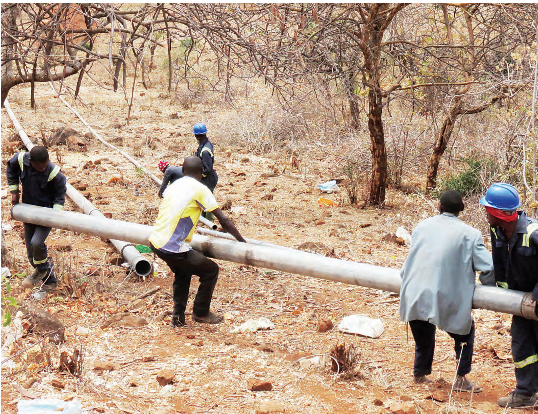
Plumbers from Kondoa-based Miraji Mgogo Ltd lay clean and safe water pipes earlier this week pending connection to tanks Plasco has built at Dabalo village in Chamwino District, Dodoma Region. Photo: Correspondent Peter Mkwavila
