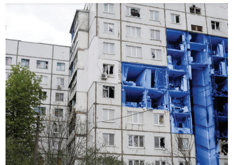
Damaged building sections in Kyiv
