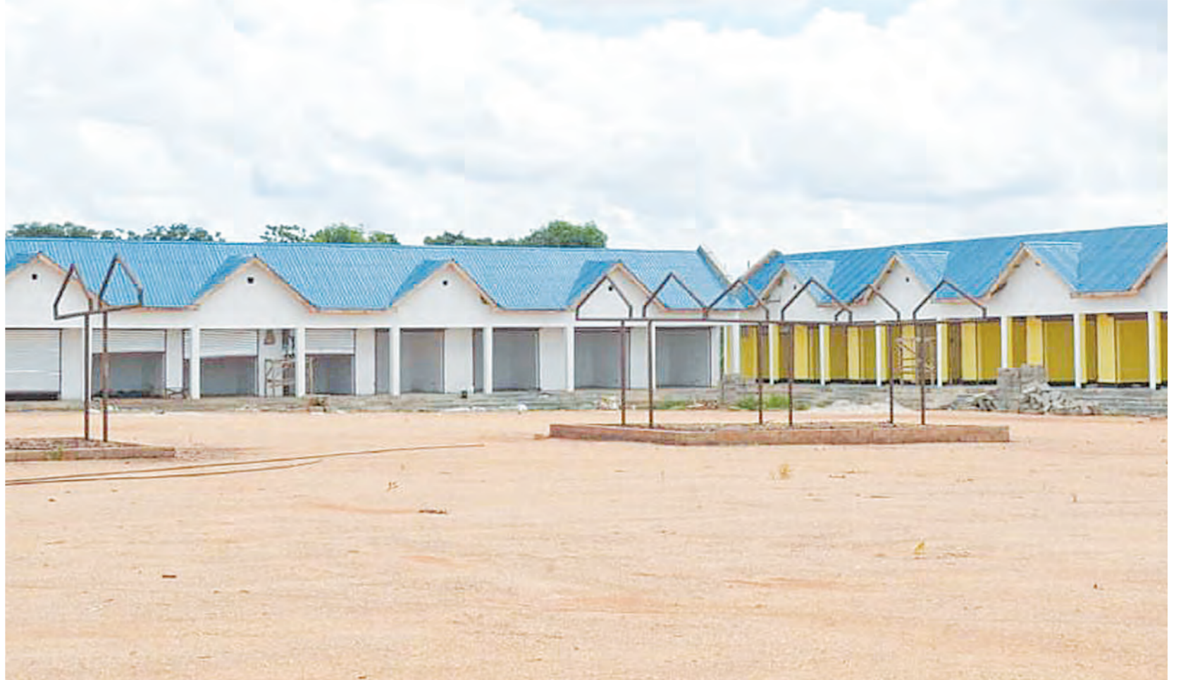
A side view of a bus terminal under construction at Lundusi village in Songea District. Photo: Francis Kajubi.
