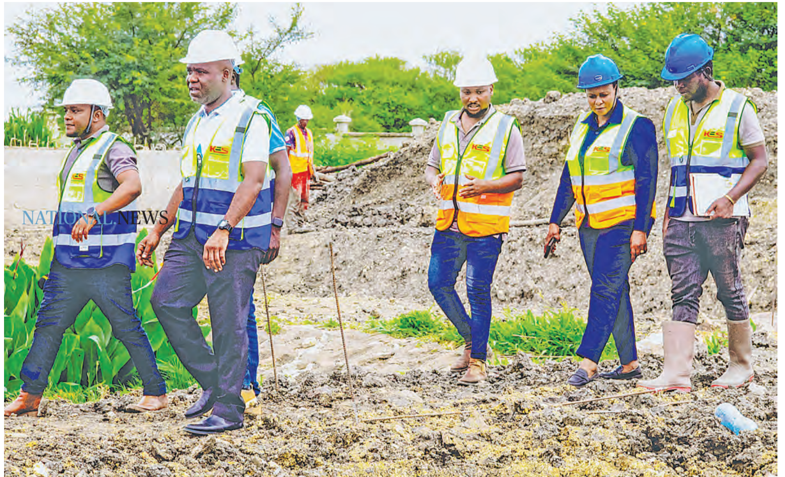
Shinyanga Urban Water Supply and Sanitation Authority executive director Yusuph Katopola (R) leads late last week's inspection of progress in the expansion of a sewage treatment plant, the idea being to serve Shinyanga municipality doubly efficiently. Photo: Correspondent Marco Maduhu
