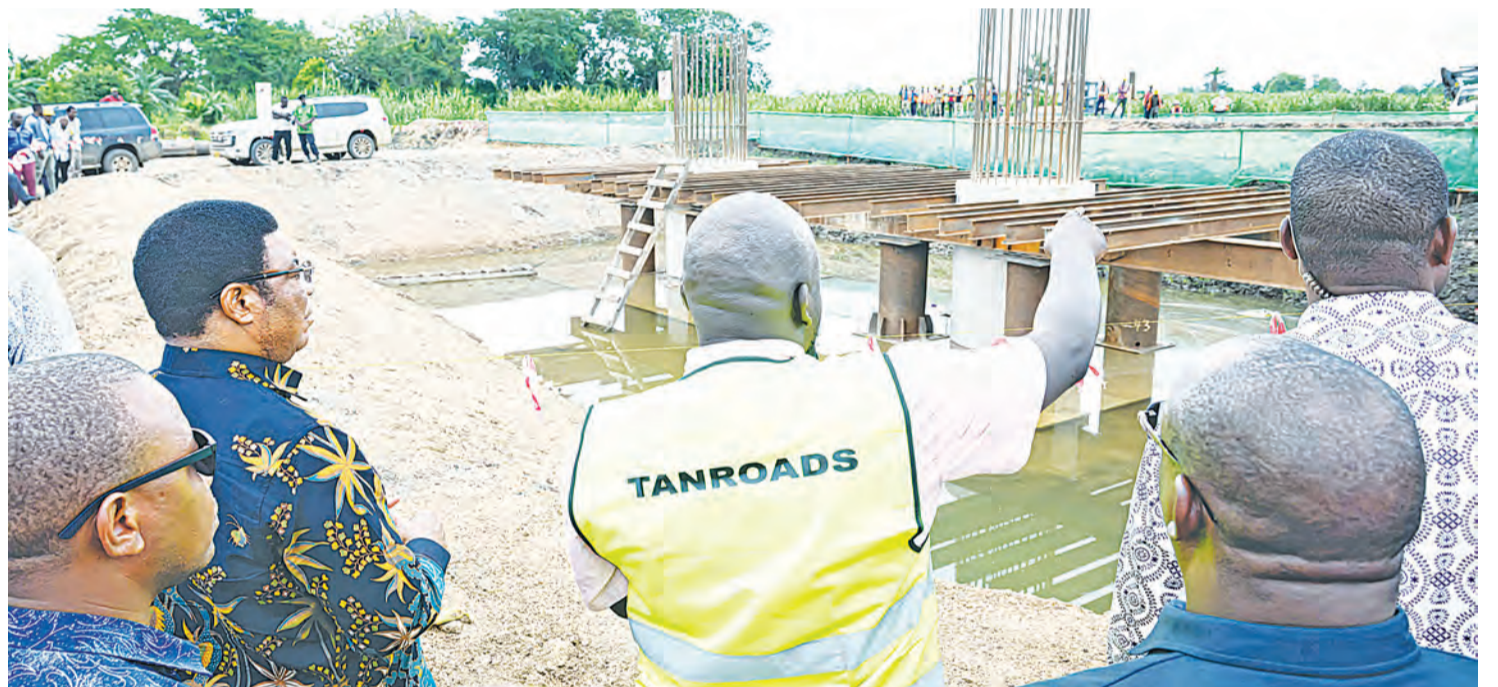
Prime Minister Kassim Majaliwa pictured yesterday while on an inspection tour of progress in the reconstruction of Simiyu Bridge, a strategic link for Mwanza, Simiyu and Mara regions. The work is expected to cost 48.7 billion/-. Photo: PMO
