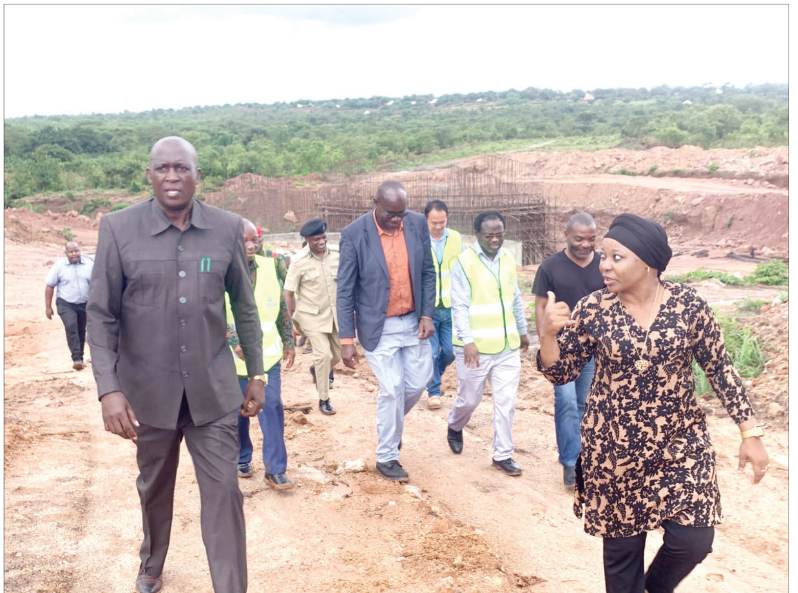
A delegation led by Ruvuma regional commissioner Col Laban Thomas (L) makes an inspection tour of the Amanimakoro-Ruanda section of a road construction project in Mbinga District yesterday. Right is Mbinga district commissioner Aziza Mangosongo. Photo: Guardian Correspondent
