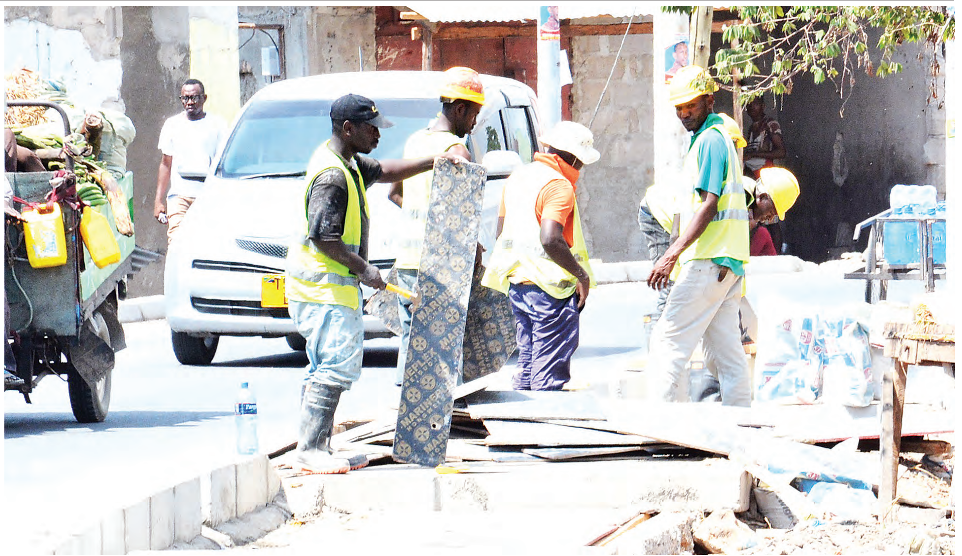
Work on a drainage system in progress along in Dar es Salaam's Tandale suburb yesterday. Photo: Correspondent Miraji Msala
