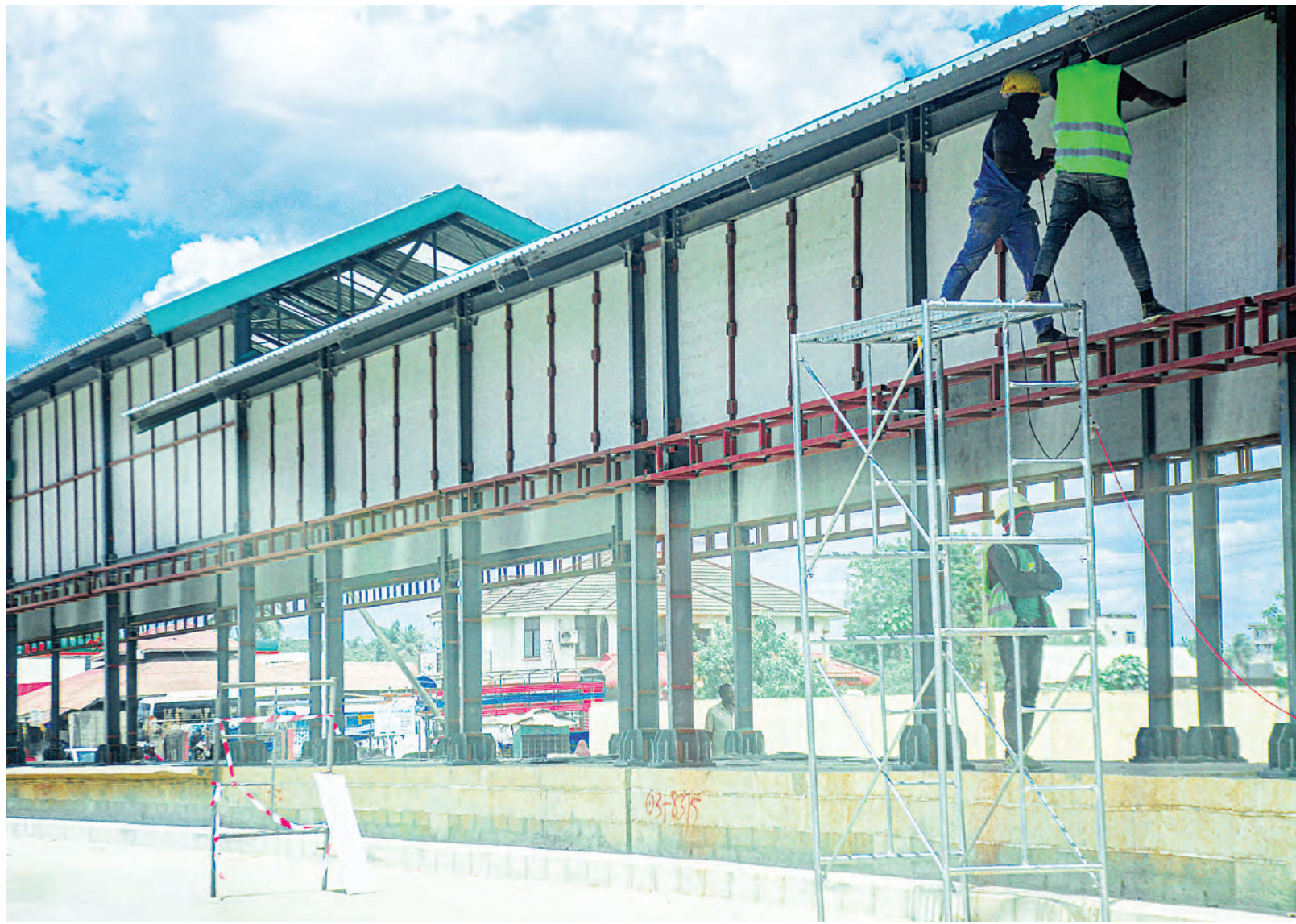
Work on a Bus rapid transit (BRT) station at the Mtoni Mtongani section of Dar es Salaam's Kilwa Road has reached an advanced stage, as confirmed yesterday. Photo: Correspondent Jumanne Juma
