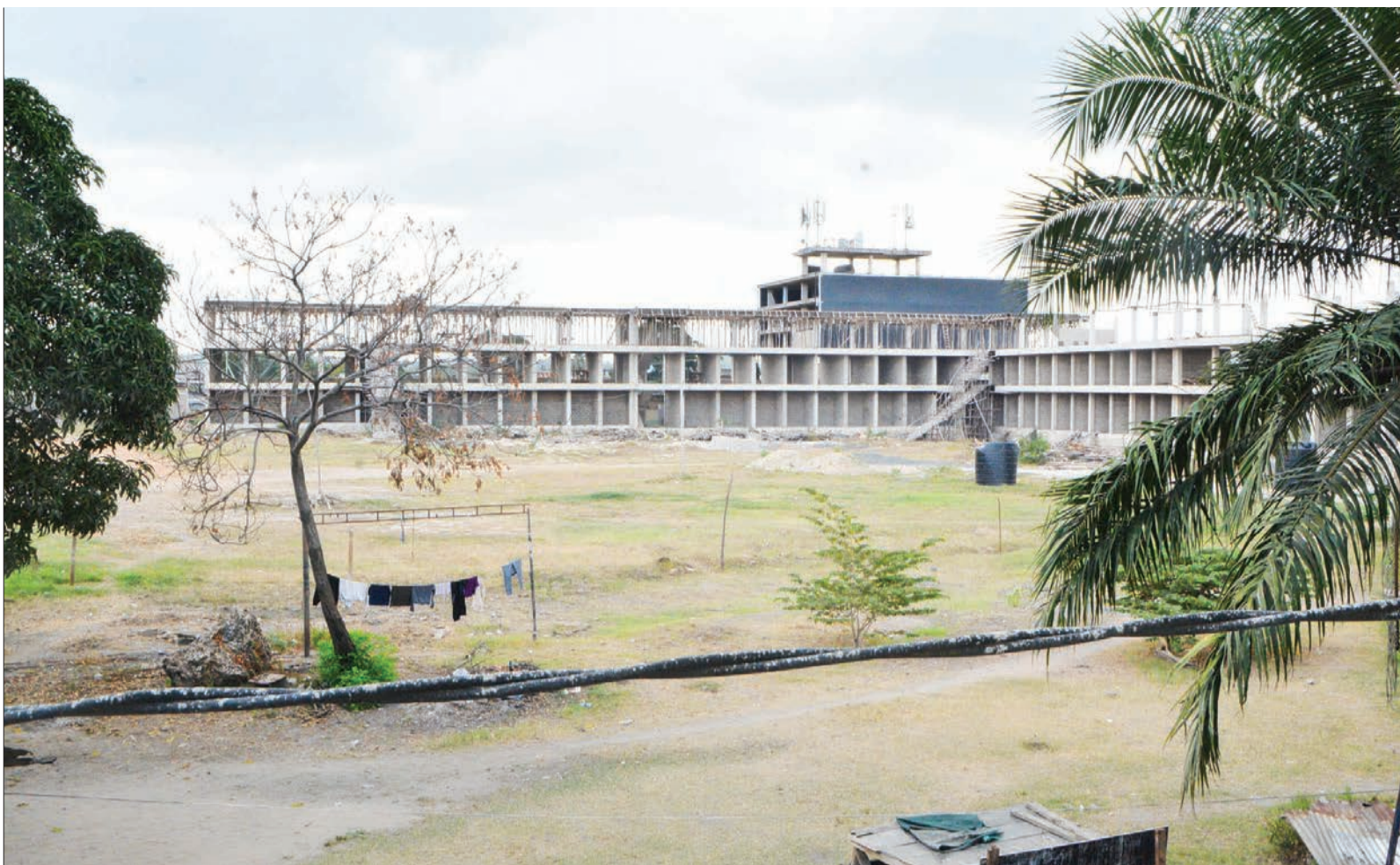
This ought to have long graduated into a modern commuter bus stand at Mwenge in Kinondoni District, Dar es Salaam. However, the project has stalled, with sources saying implementation is expected to resume only after reported differences of opinion between the contractor and the Kinondoni Municipal Council are resolved. Photo: Correspondent Miraji Msala
