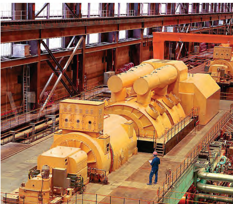
A Steam driven turbine in power station with supervisor. Photo: Courtesy of Mira Image
