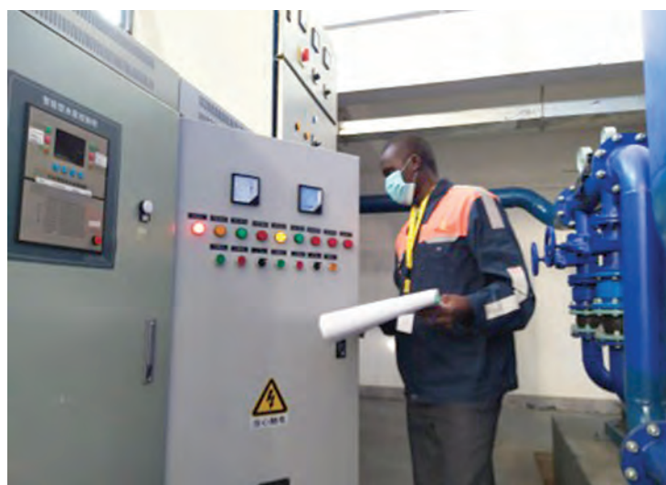
A local electrician checks the equipment at a plant along the Mombasa-Nairobi standard gauge railway. (File photo)
