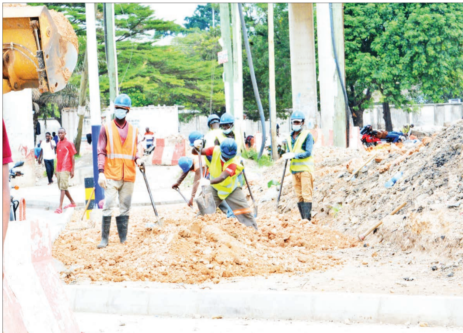
Preparations for the construction of a sidewalk in progress at Ubungu in Dar es Salaam yesterday. Photo: Correspondent Miraji Msala
