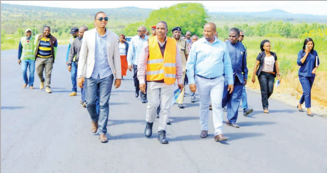
Iringa regional commissioner Ally Hapi (L, foreground), Iringa's Tanzania National Roads Agency (Tanroads) regional manager Daniel Kindole (C) and Iringa Municipal mayor Ibrahim Ngwada (R) pictured yesterday having an eyewitness account of the implementation of the project involving the expansion of Iringa Airport. Photo: Correspondent Friday Simbaya
