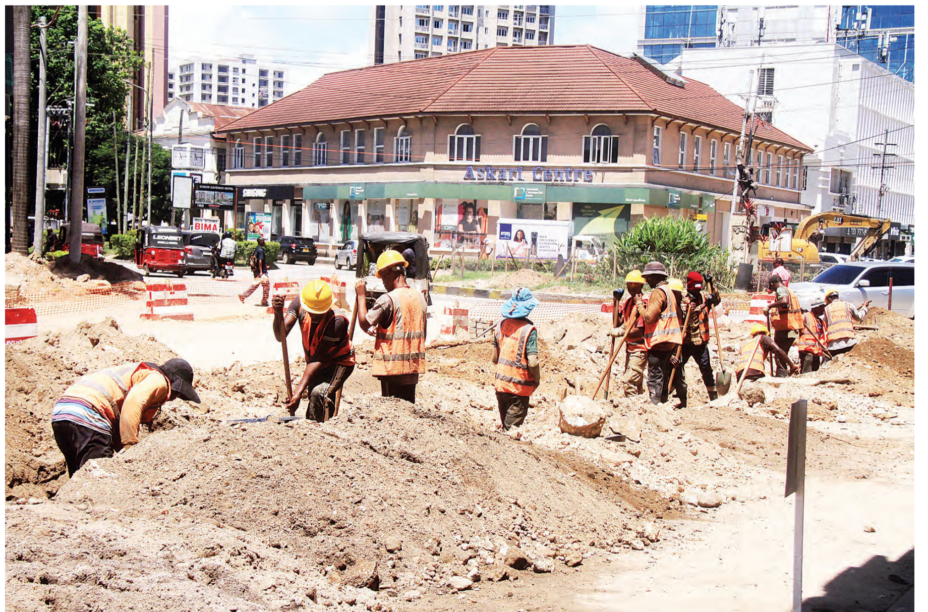
Sinohydro Construction Company workers dig a trench as part of the ongoing implementation of the rapid bus road infrastructure project along Azikiwe Road in downtown Dar es Salaam yesterday. Photo: Correspondent Jumanne Juma
