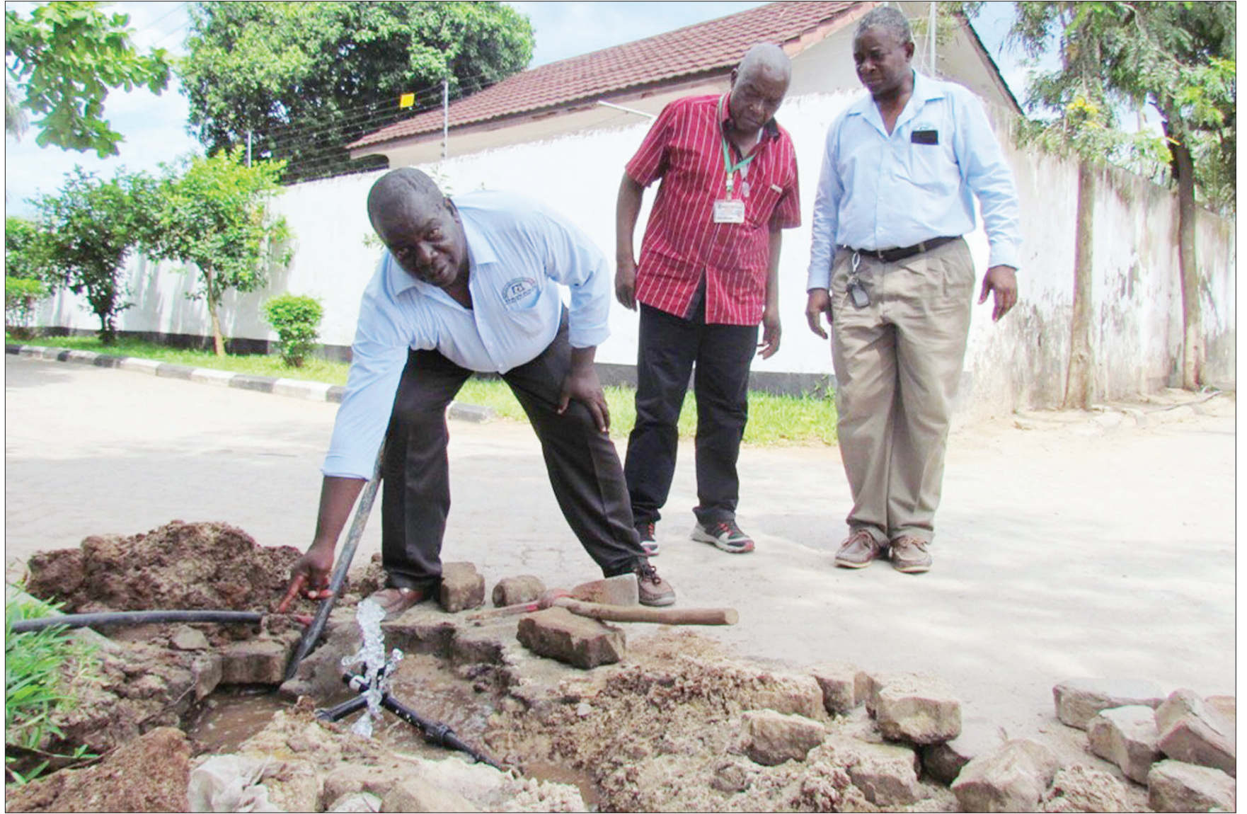
Dar es Salaam Water and Sewerage Authority meter reader Mohamed Mwakimila (L) pictured along Muzimuni Street in the city's Kawe suburb yesterday pointing at a water pipe said to be illegally connected to a bigger one, as a nationwide operation meant to arrest the trend continues. Photo: Guardian Correspondent
