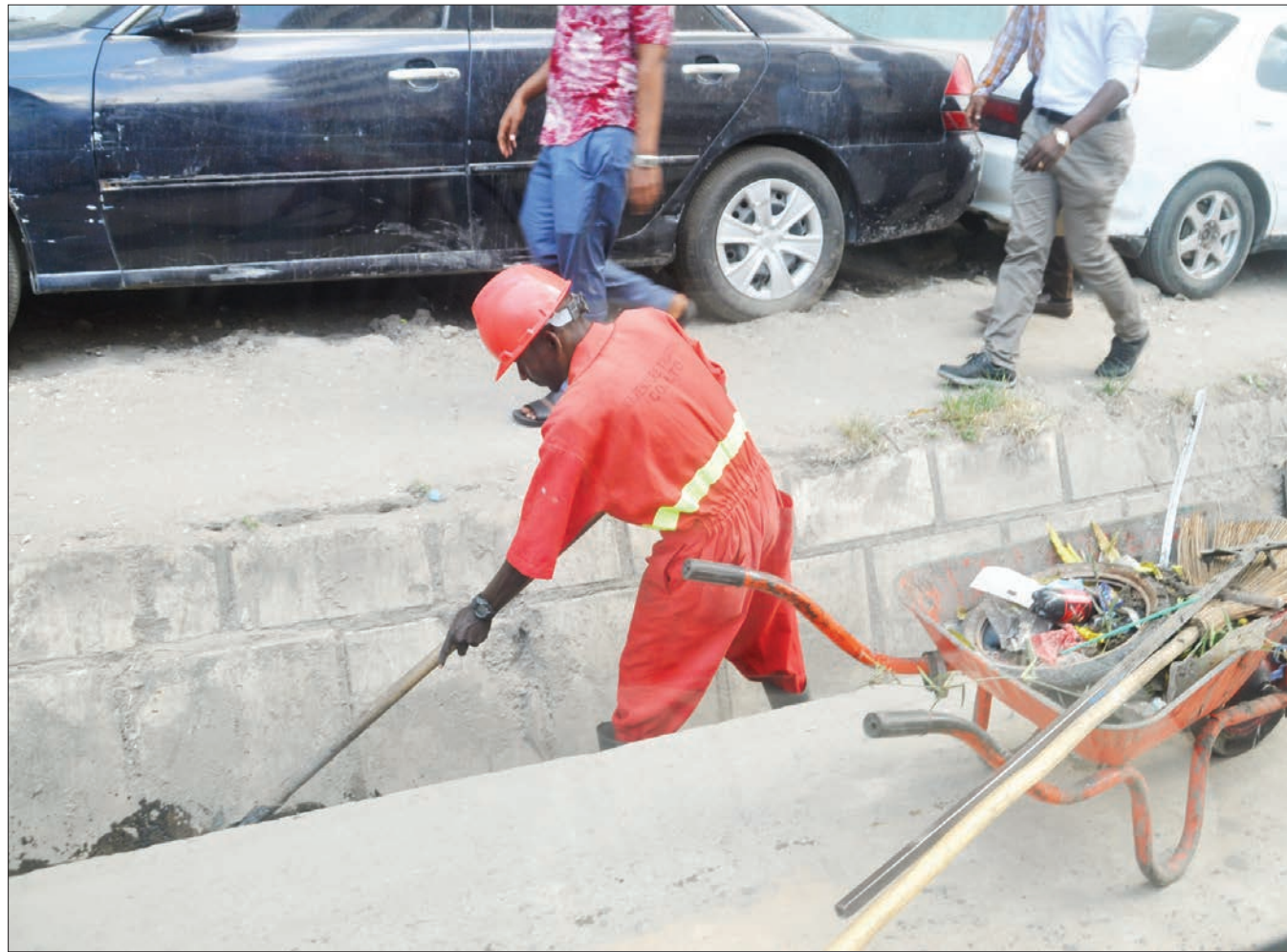
Clearing of a drainage system gets under way yesterday along Muheza Street in Dar es Salaam city's sprawling Kariakoo market area. Photo: John Badi
