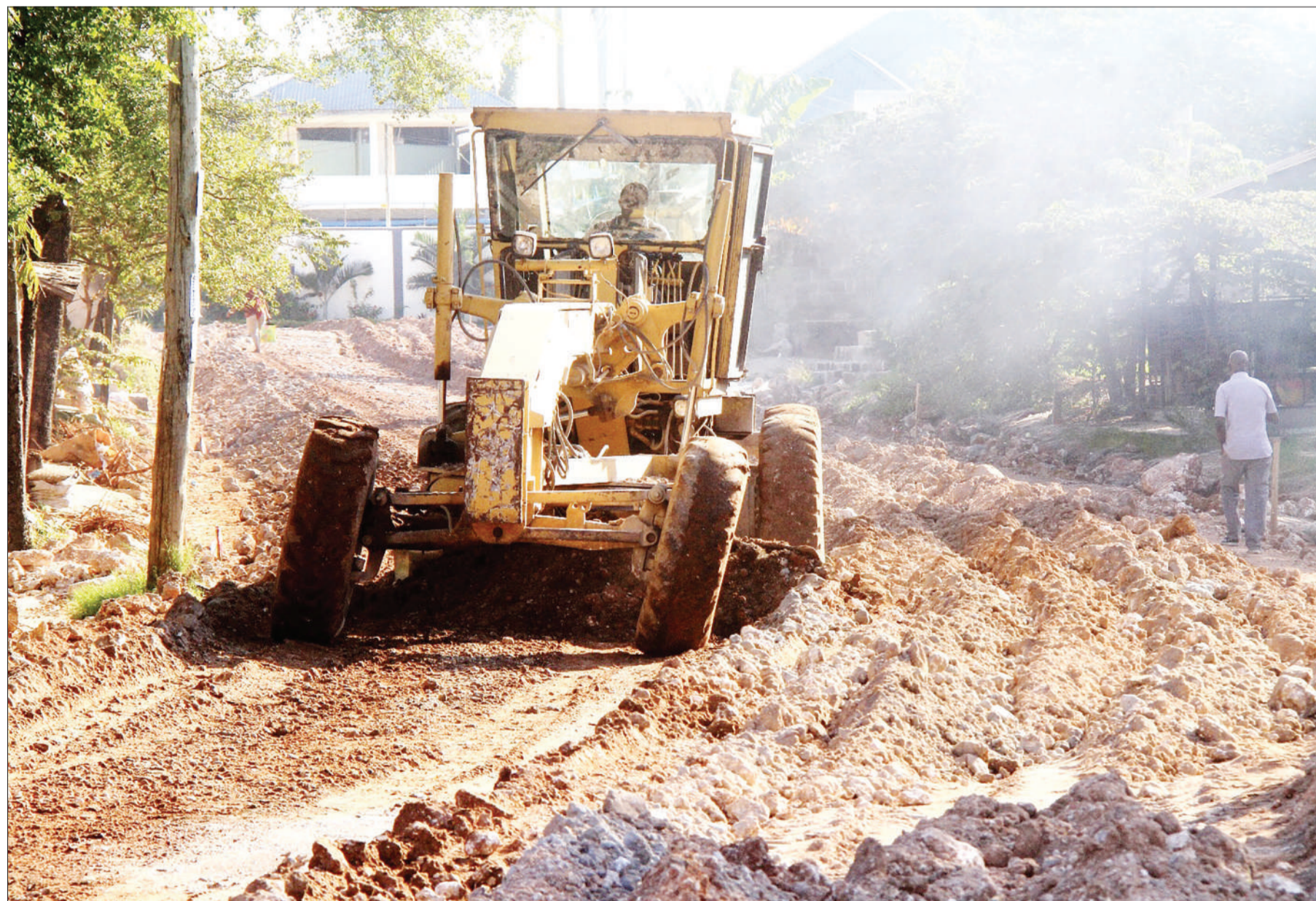
A grader levels a stretch of an unpaved road in Dar es Salaam's Kitunda Machimbo suburb yesterday pending its tarmacking. Photo: Correspondent Jumanne Juma
