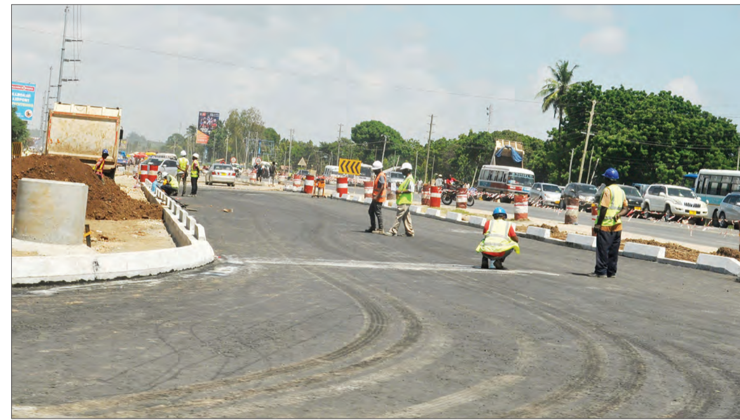
Workers with heavy construction equipment making progress in expansion of the New Bagamoyo Road to four ways from Morocco to Mwenge at Kijitonyama-Science area in Dar es Salaam yesterday. Photo: John Badi.
